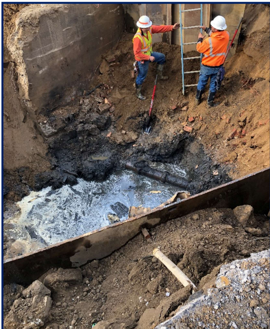
Fig 2: Water uncovered during excavation
