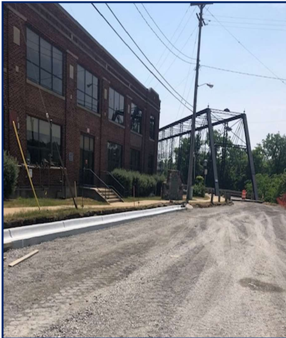
Fig 2: Duran Concrete begins placement of new curb and gutter along 2nd St and Brady St.
