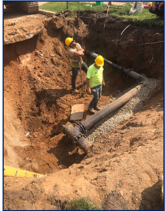
Fig 1: Milbocker's pipe crew ties the water main on Hubbard St into Chestnut St.
