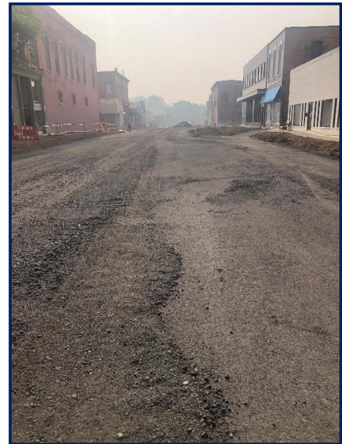
Fig 1: Milbocker continues to build up the road base along E Hubbard St in preparation for curb and asphalt
