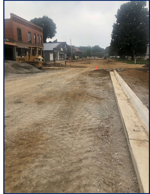
Fig 1: Milbocker finalizes road grades to prepare for asphalt paving in the coming weeks.
