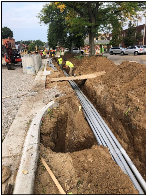
Fig 2: Severance Electric continues to install conduits ahead of sidewalk and grading crews to allow for underground utilities.
