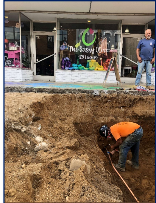
Fig 1: Milbocker works to finish installation of water services to various properties on Locust St
