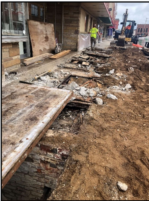
Fig 2: Basements underneath the sidewalk on Locust St are abandoned
