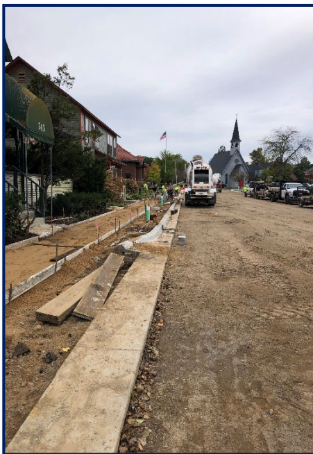
Figure 2: Roadway along Hubbard Street being prepared for the installation of curb and sidewalks.
