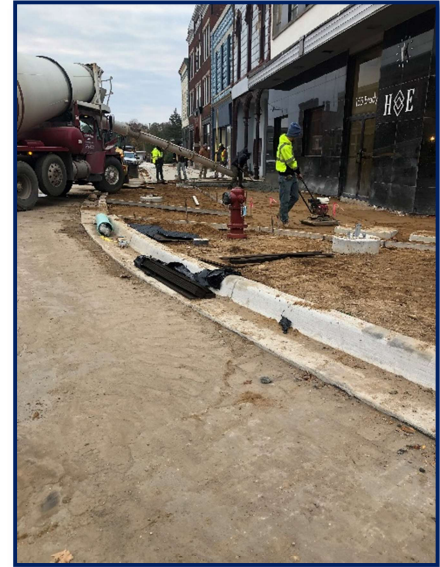
Figure 1: Duran and Milbocker work together to grade and pour concrete in front of Hartman-Ellis Agency.
