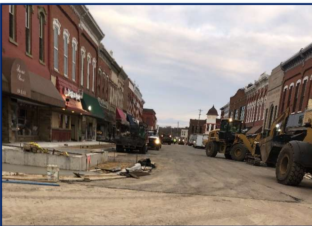
Figure 2: Construction equipment moves onto Locust St. after base course paving to prepare for continued concrete work on Locust St.
