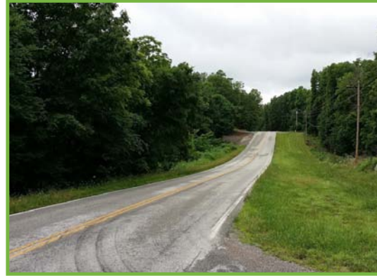
Wide shoulder along Hampstead Rd. near Winters Dr. provides adequate width and grade for a shared use trail.
