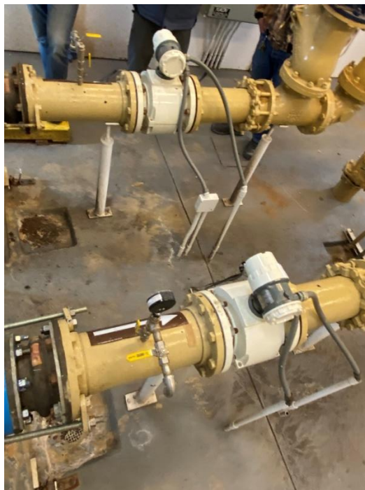
WASTE ACTIVATED SLUDGE FLOW METER FROM EACH PUMP
