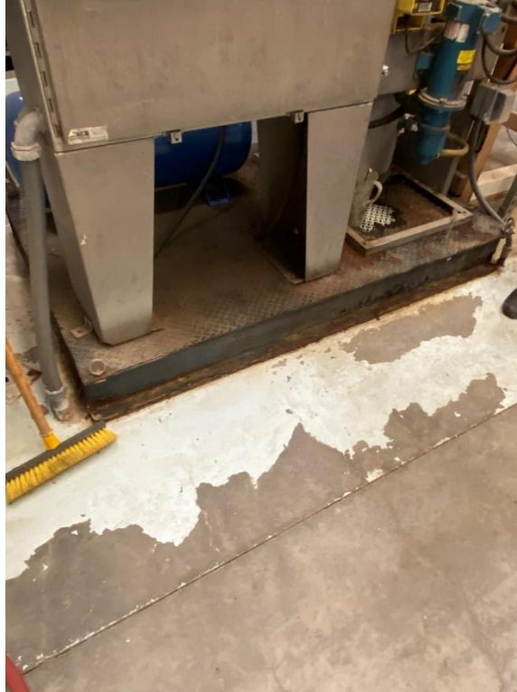
POLYMER UNIT METAL BASE IS CORRODED
