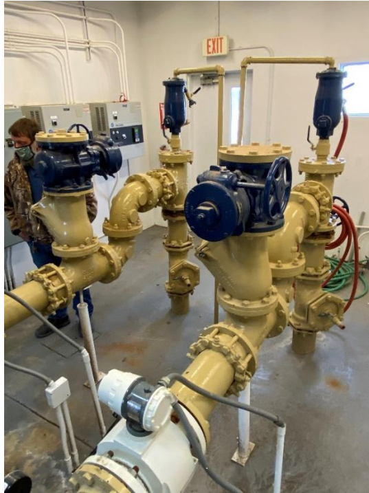
WASTE ACTIVATED SLUDGE PUMPS DISCHARGE TO BELT FILTER PRESS
