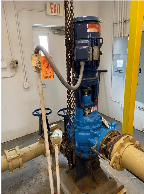
WASTE ACTIVATED SLUDGE PUMP NO. 1 – FEED TO BELT FILTER PRESS
