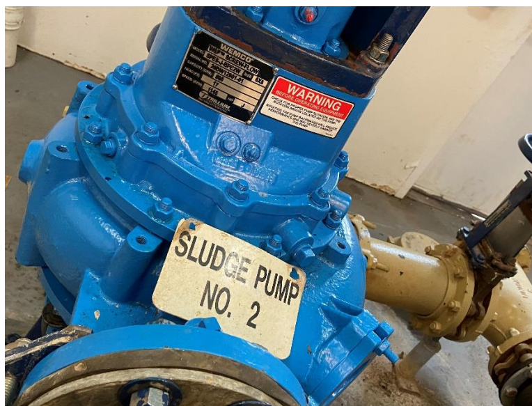
WASTE ACTIVATED SLUDGE PUMPS - RECENTLY REPLACED
