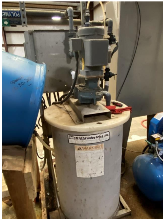
POLYMER MIXER AND MIX TANK
