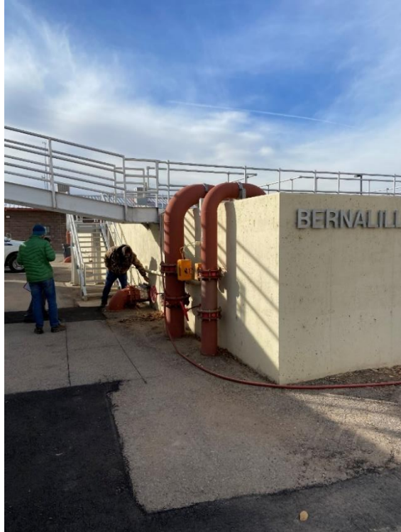
LEAK THROUGH EAST WALL OF STURCTURE AT INLET PIPE
