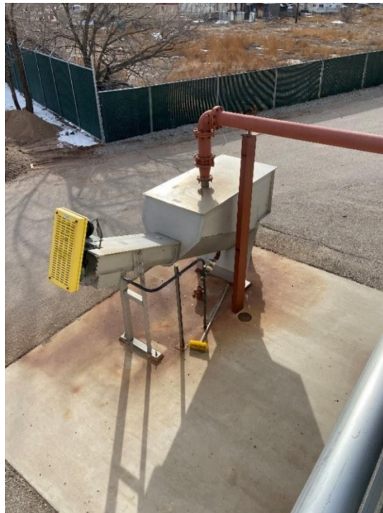
HYDROGRITTER DOES NOT FULLY FUNCTION DUE TO POOR PREFORMANCE FROM AIR LIFT PUMPS IN AERATED GRIT CHAMBER
