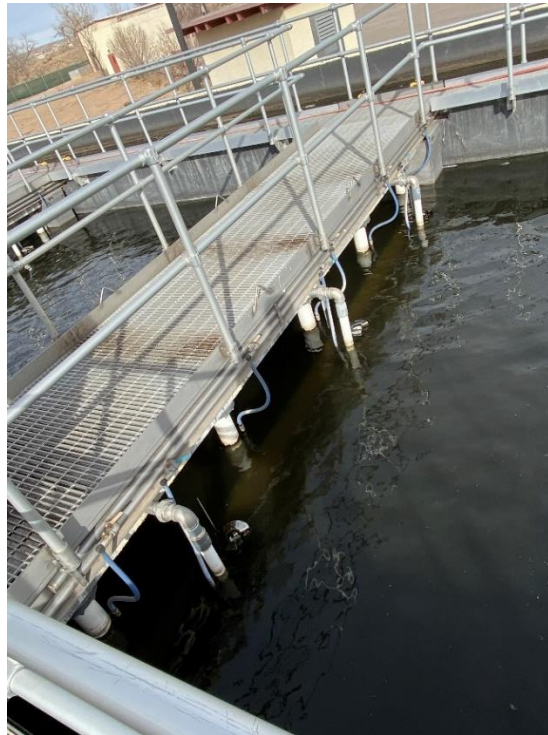
VIEW OF CLARIFIER BRIDGE WITH AIR SUPPLY TO SUBMERGED SKIMMERS
