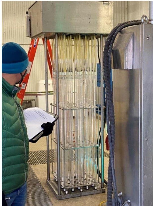
UV BULBS NEEDING REPLACEMENT (LIFTED OUT OF CHANNEL)
