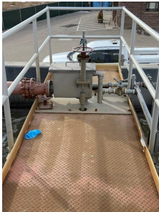
STEEL PLATFORM ABOVE AERATED GRIT CHAMBER IS RUSTED AND CORRODED
