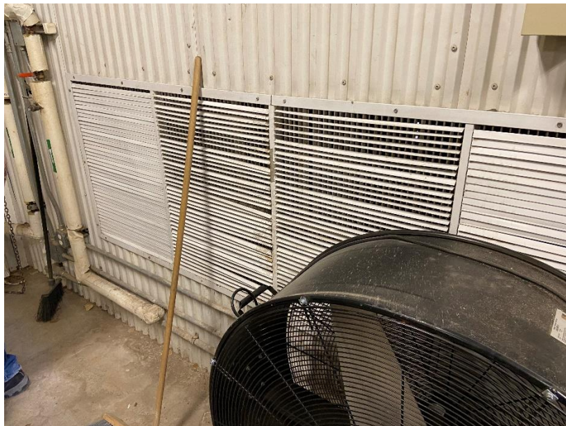
WATER SPRAYS THROUGH LOUVER FROM SOUTH COOLER UNIT THROUGH WALL INTO BUILDING AND BLOWER ENCLOSURE
