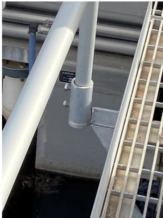
BROKEN WELDED CONNECTION ON HANDRAIL POST BRACKET
