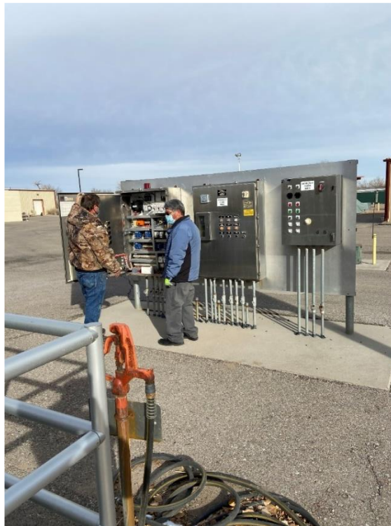
EXISTING INFLUENT PUMP STATION CONTROL PANELS
