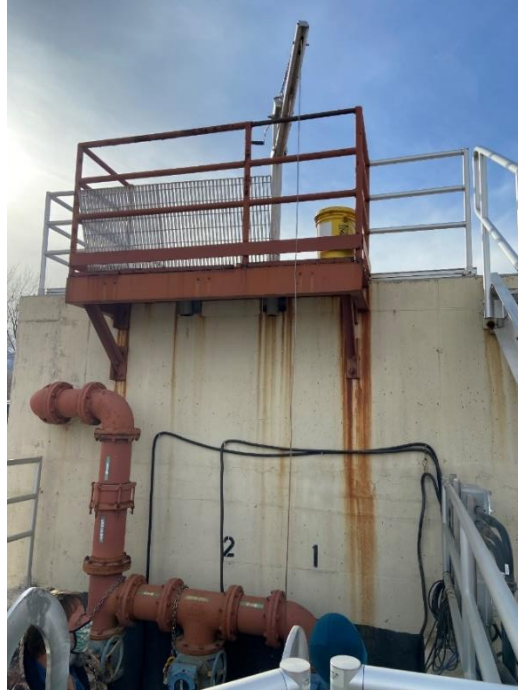
CORRODED STEEL PLATFORM AND HANDRAIL ABOVE WET WELL
