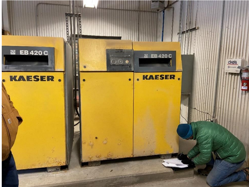
BLOWER ENCLOSURE CORRODING FROM OVER SPRAY FROM SOUTH COOLER UNIT THROUGH WALL
