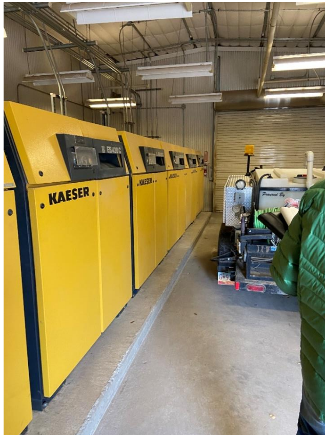
VIEW OF BLOWER UNITS ON HOUSER PAD
