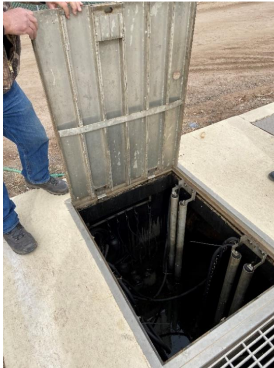
WET WELL PUMP COVER (NO FALL PROTECTION)
