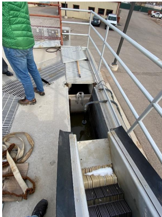
SLIDE PLATES DO NOT EFFECTIVELY SHUTOFF FLOW IN SCREENING CHANNEL IN CLOSED POSITION. MECHANICAL STAIR SCREEN STEPS ICE UP.
