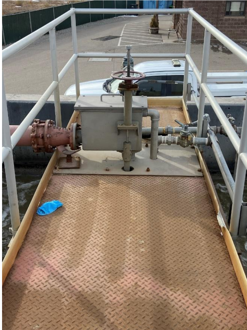
RUSTED STEEL PLATFORM ABOVE AERATED GRIT CHAMBER
