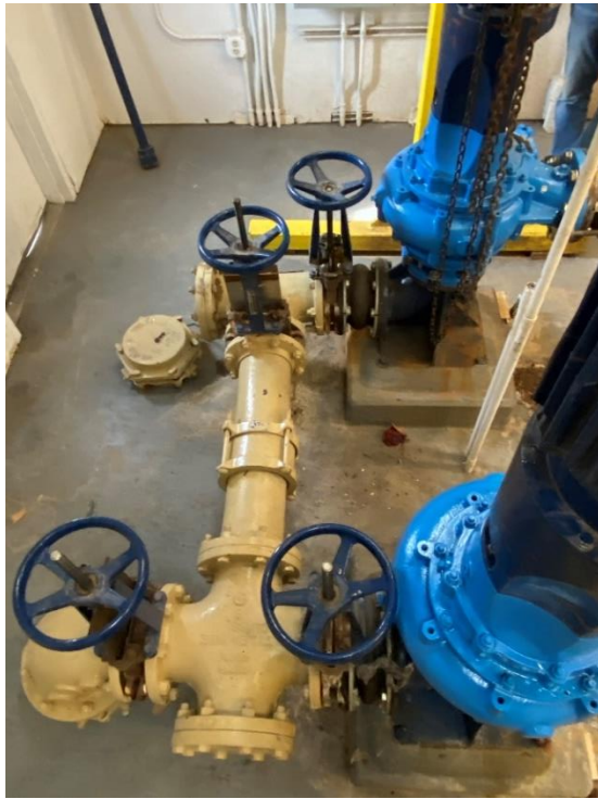
WASTE ACTIVATED SLUDGE SUCTION TO PUMP SUPPLY SOURCE FROM AEROBIC DIGESTER
