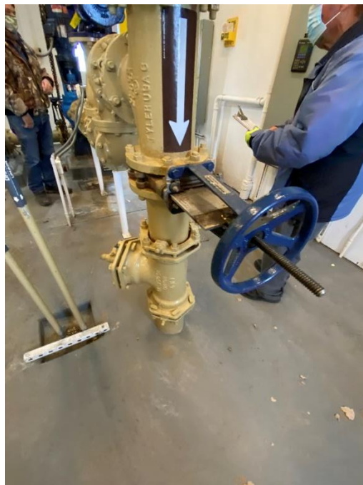
WASTE ACTIVATED SLUDGE DISCHARGE PIPING WITH KNIFE GATE VALVES
