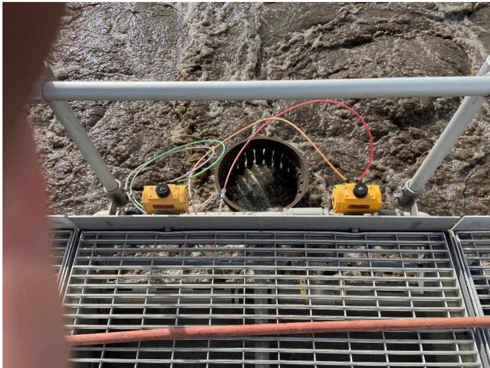
AIR ACTUATOR PLASTIC TUBE LINES ARE NOT ULTRAVIOLET RESISTANT
