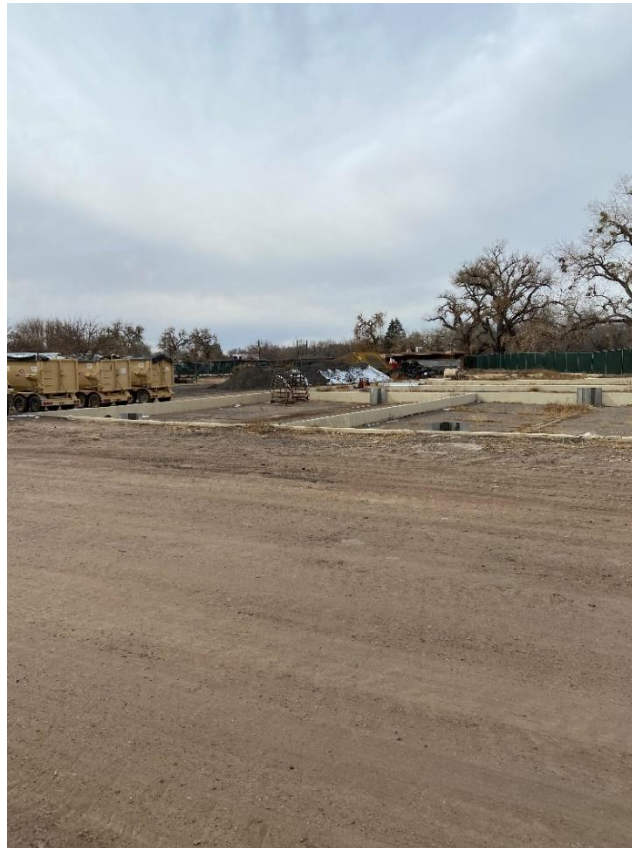
SLUDGE DRYING BEDS – WEST END
