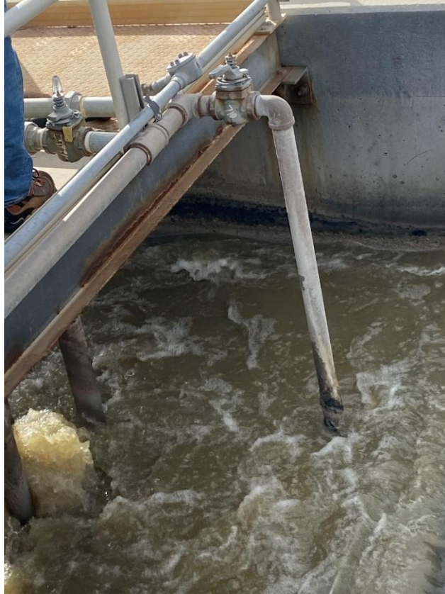
STEEL STRUCTURAL MEMBERS ARE CORRODED
