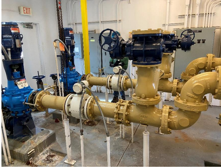
WASTE ACTIVATED SLUDGE PUMPS AND DISCHARGE PIPING WITH FLOW METER
