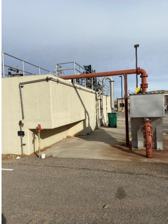
MECHANICAL STAIR SCREEN ON TOP OF STRUCTURE WITH WASH PRESS AND SIDE DISCHARGE CHUTE TO DUMP CONTAINER ON GROUND LEVEL
