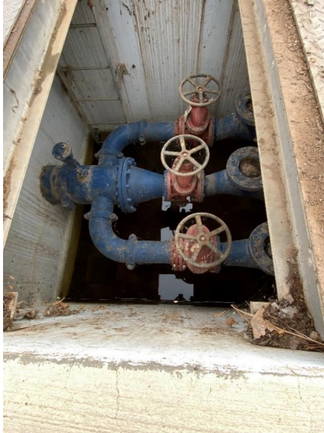
RAINWATER IN VALVE PIT
