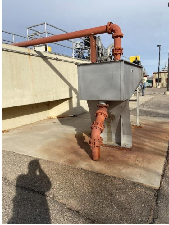
HYDROGRITTER – FREEZING CONDITIONS CAUSE OPERATIONAL PROBLEMS AND SHUTDOWN OF UNIT DURING WINTER OPERATIONS\
