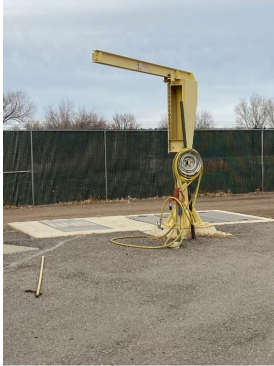
EFFLUENT LIFT STATION WITH JIB CRANE FOR PUMP REMOVAL
