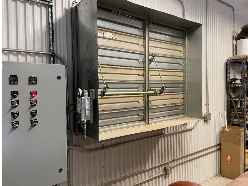
MOTORIZED WALL LOUVERS - ACTUATOR NOT WORKING PROPERLY
