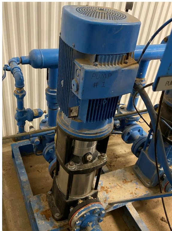
WASHWATER BOOSTER PUMP ON SKID FRAME
