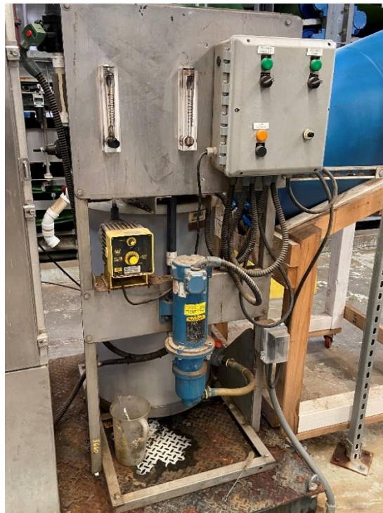
POLYMER PANEL WITH MOUNTED METERING PUMP AND ELECTRICAL CONTROL PANEL
