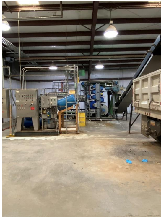
EAST VIEW OF POLYMER SYSTEM AND BELT FILTER PRESS AREA IN BUILDING
