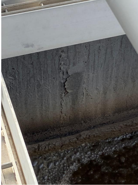
VIEW OF DELAMINATION OCCURING IN AEROBIC DIGESTER BASINS
