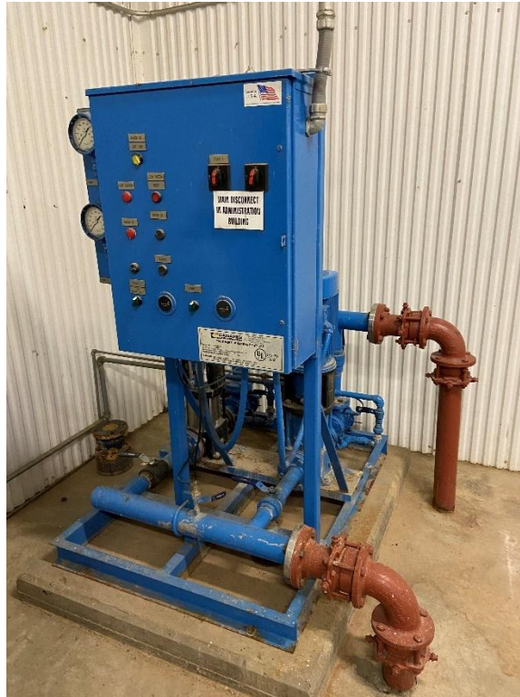
WASHWATER BOOSTER PUMP STATION – SKID MOUNTED
