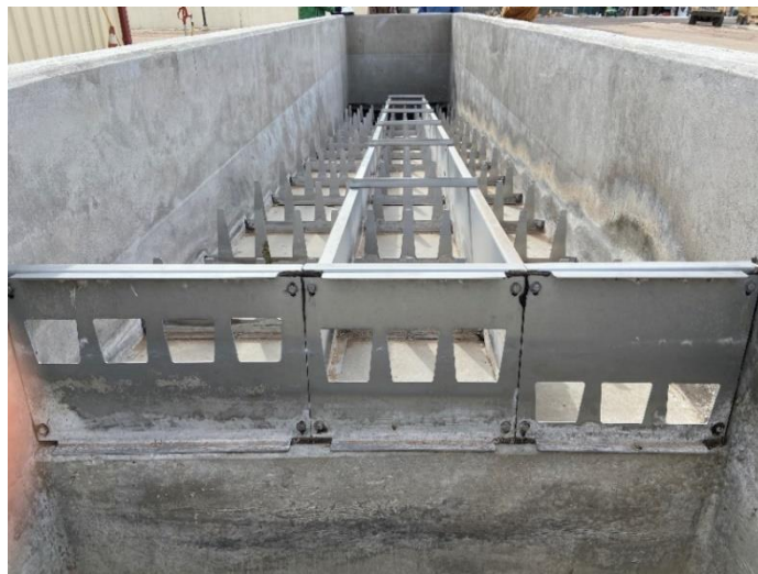
CASCADE AERATOR STRUCTURE AND FLOW CONTROL PLATES WITH AERATION FINGERS TO OUTLET BOX
