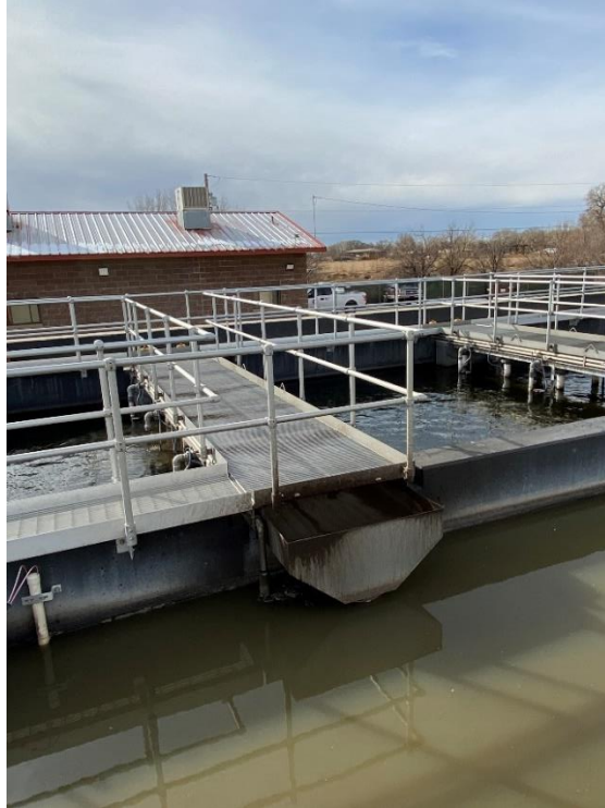
VIEW OF CLARIFIER WALKWAY BRIDGE WITH RAS TROUGH UNDER BRIDGE TO FERMENTER BASIN
