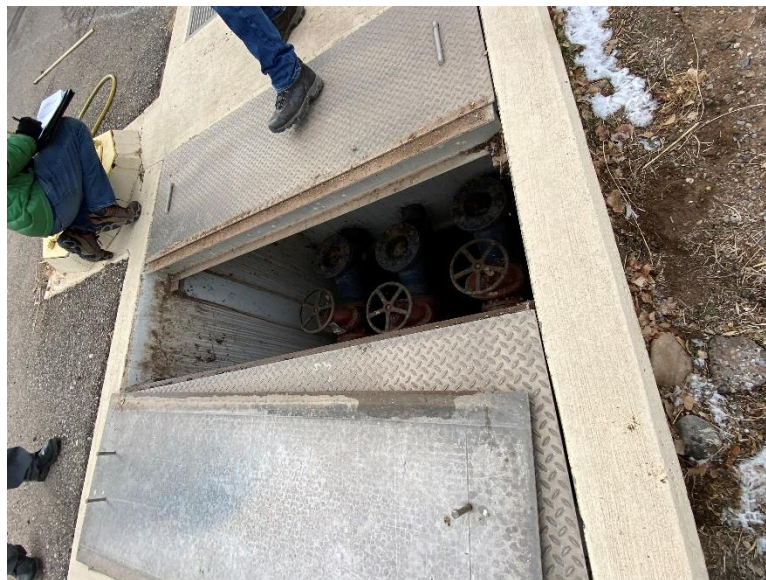
VALVE PIT COVER WITHOUT FALL PROTECTION
