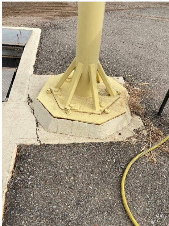
JIB CRANE - BROKEN CONCRETE BASE
