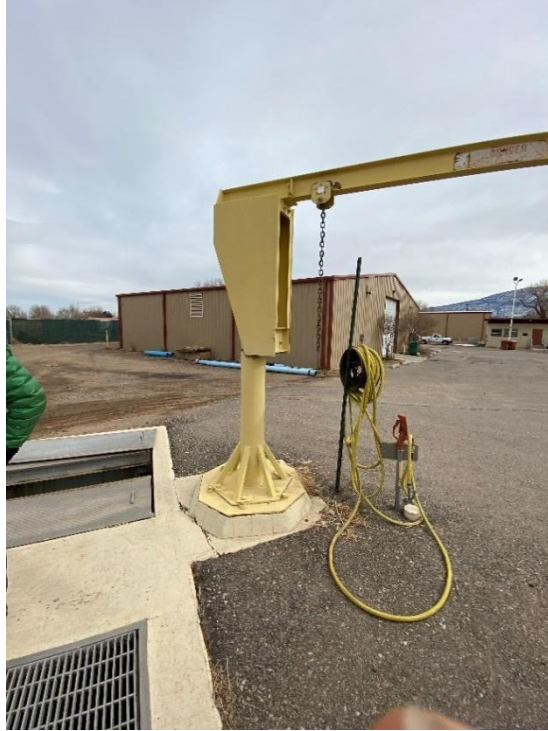
VIEW OF JIB CRANE AT LIFT STATION
