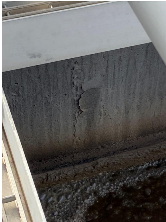
EXAMPLE OF DELAMINATING COATING ON BASIN WALLS
