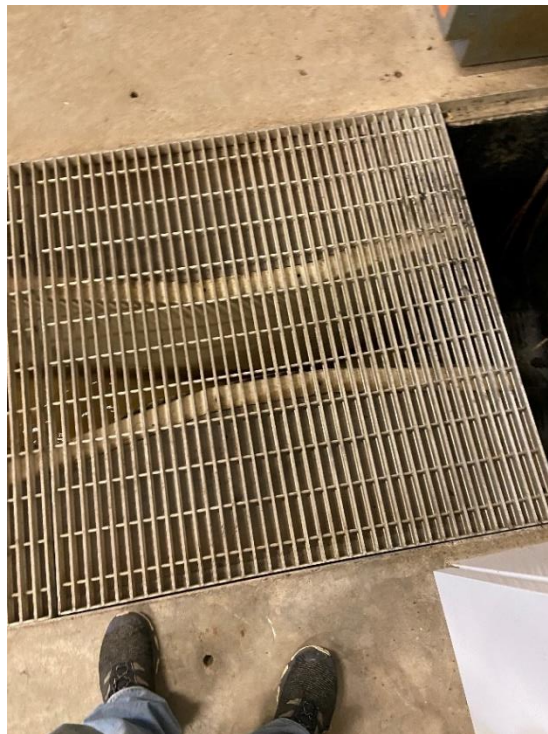
VIEW OF PARSHALL FLUME IN CHANNEL
