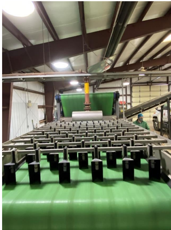
BELT FILTER PRESS BELT TOP BELT WITH WEDGES FOR DISTRIBUTION OF FEED SLUDGE
