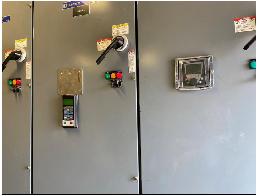
BLOWER VFD CABINETS WITH OLD VFD UNIT AND REPLACED VFD UNIT
