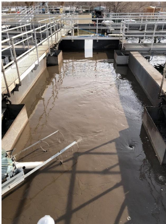
ANAEROBIC SELECTOR BASIN WITH MIXER
