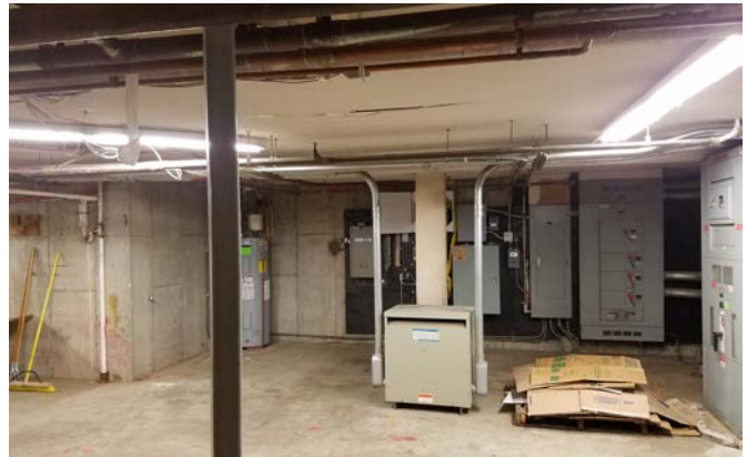
58. Basement Electrical Switch Gear
