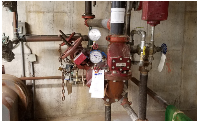
60. Basement Fire Suppression
