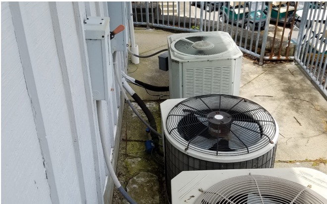
45. HVAC Condensing Units
