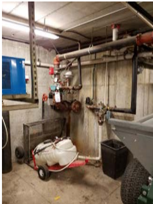
35. Fire Suppression Riser
