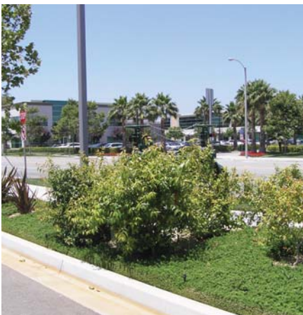
Backflow preventers should be screened with landscaping or fencing
