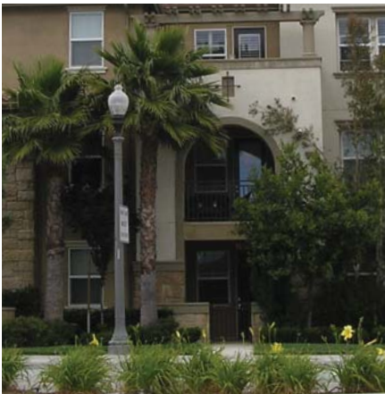
Residential light fixture
