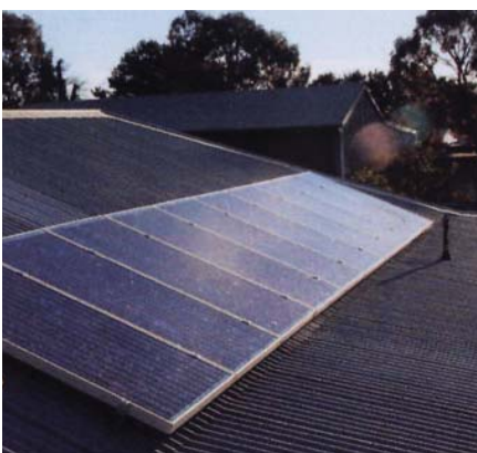
Solar panels should be screened from public view wherever possible or integrated into the roof
