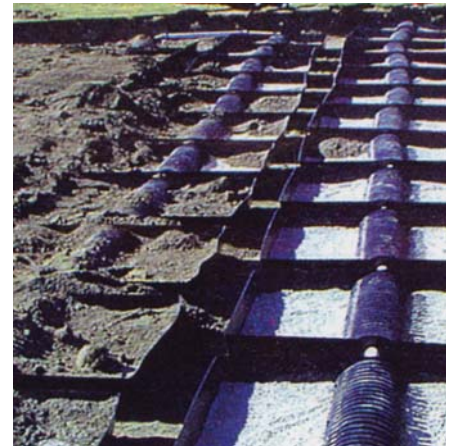
Subsurface irrigation system
