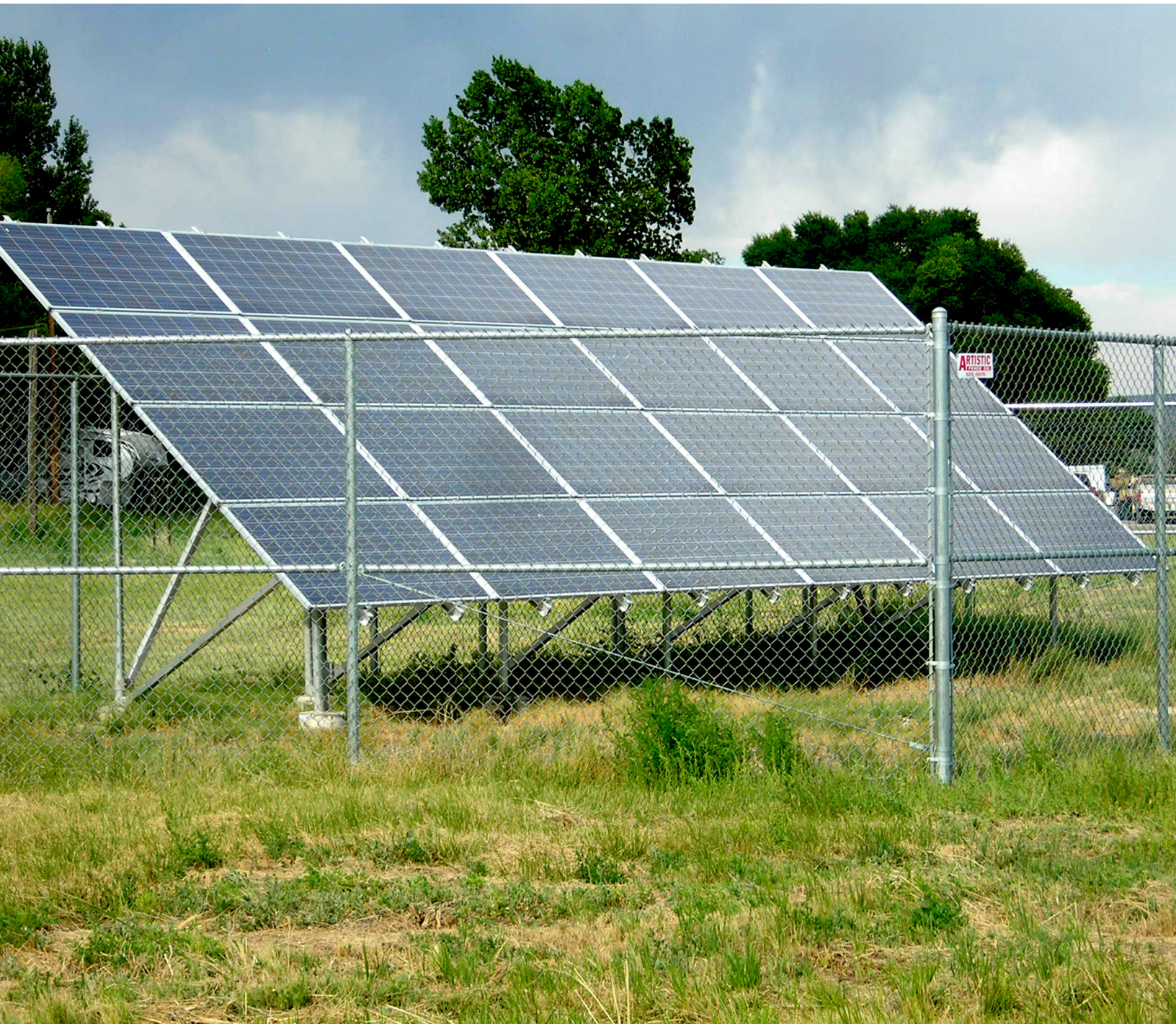
Image 23: Solar Panels, Carlin, NV. CTA (2013)
