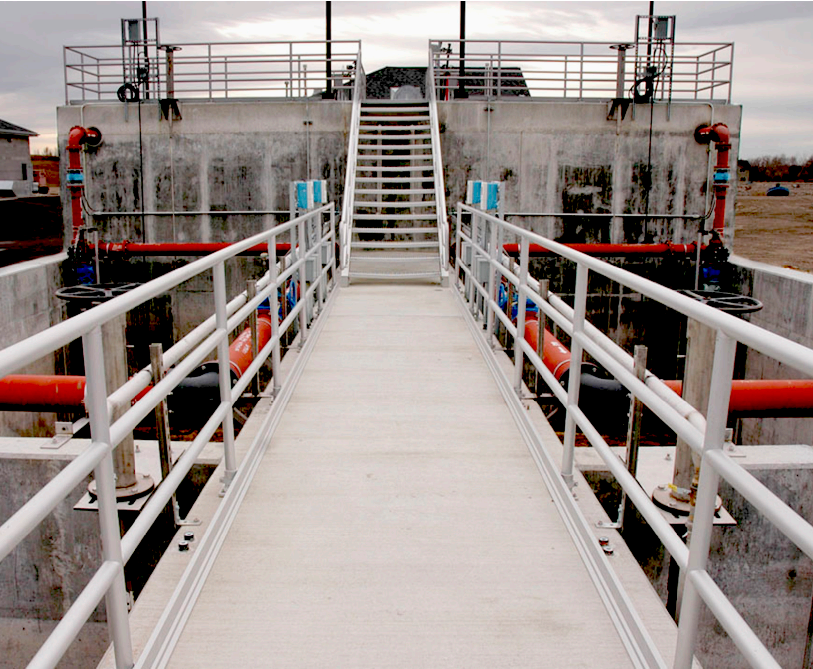
Image 24: Sanitary Sewer Treatment Facility (CTA, 2011).z
