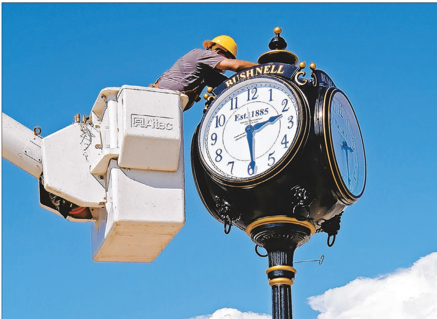
A Bushnell Public Works employee makes a final adjustment to the clock head before its anchored into place and the electrical wiring is completed.
