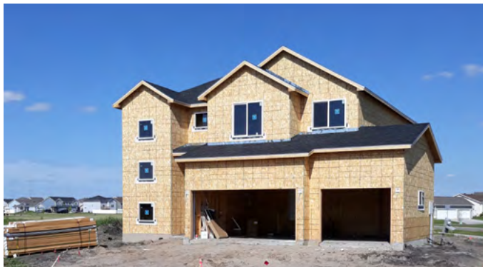
Construction of single-family residences continues to dominate redevelopment activity throughout Horace. (Source: Stantec)
