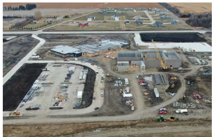
Construction of the new middle school and high school in Horace. (Source: City of Horace)
