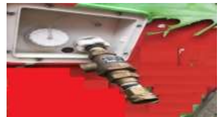
Backflow preventer installed on exterior of unit for connection of public water line
