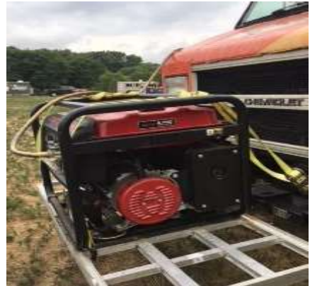
Generator installed outside of unit
