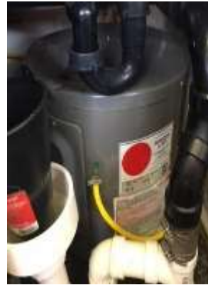
Tank water heater
