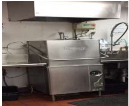
Type II hood over heat/moisture producing dishmachine
