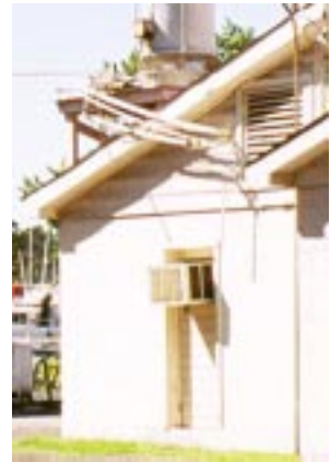
Filling in this door to house an air conditioning unit is inappropriate.
