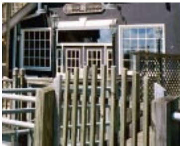
These multi-paned windows have an inappropriate snap-in grid system.
