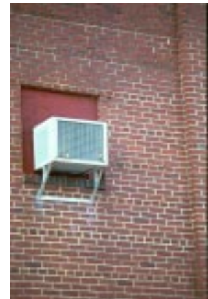
This air conditioning unit has been properly placed on the less visible side facade of the building in an existing opening.
