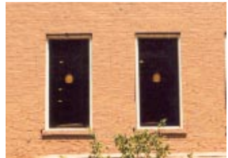
Upper floor windows on this building have been replaced with plate glass, removing all evidence of historic windowpane configuration.
