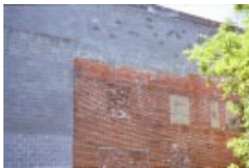
This inappropriate addition encases the original historic building, removing its innate historic character and identity.
