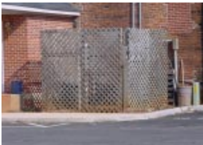
This mechanical system has been properly screened with latticework.
