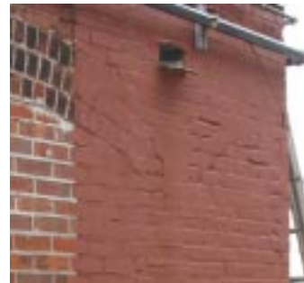
The downspout for this roof drain is missing and is causing water damage to this brick work.
