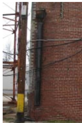
This downspout is in need of repair so that the water is directed away from the building.
