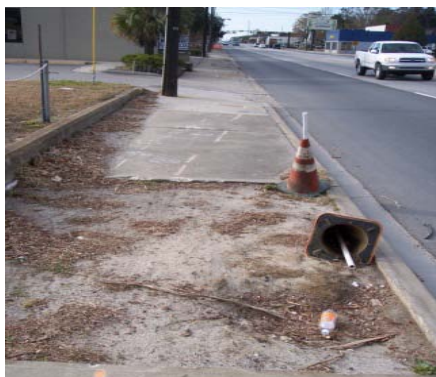
Section of South Fraser Street's sidewalk in need of repair
