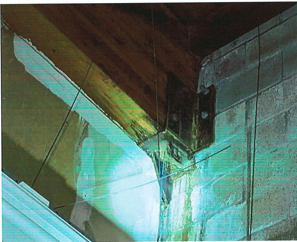
Photo 26 – Glulam beam deterioration at toe, Building C
