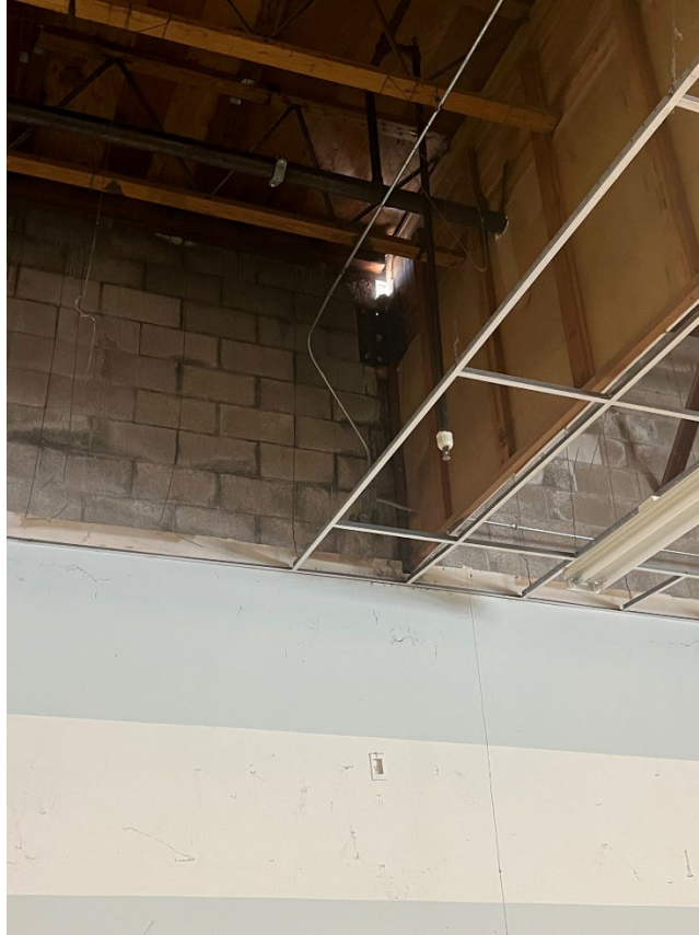
Unit C – Holes in shared wall with Unit B, exposing structural elements to weather exposure since initial roof collapse
