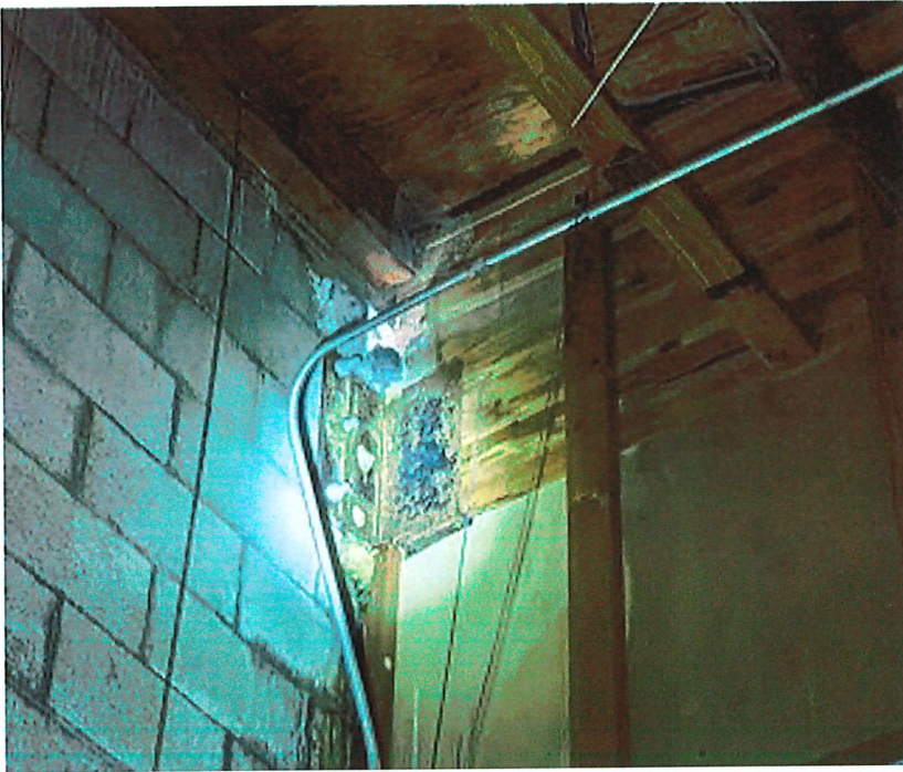
Photo 25 – Visible daylight behind deteriorated glulam beam, Building C
