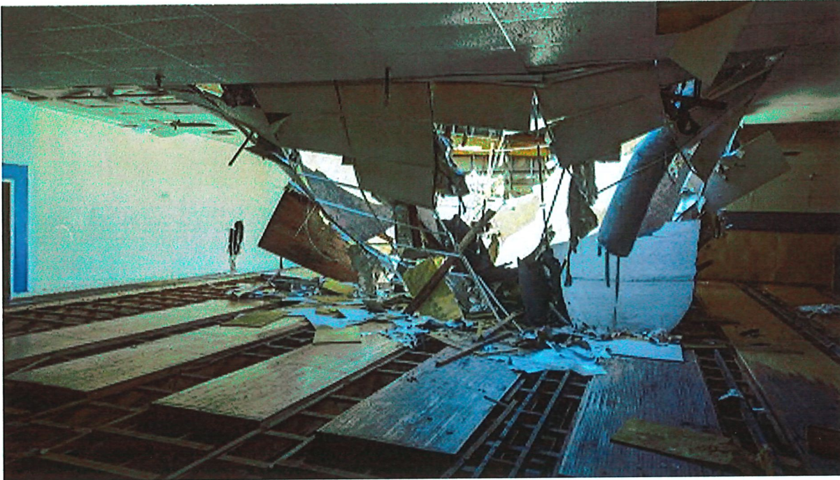
Photo 1 – Collapsed Roof, Building A
