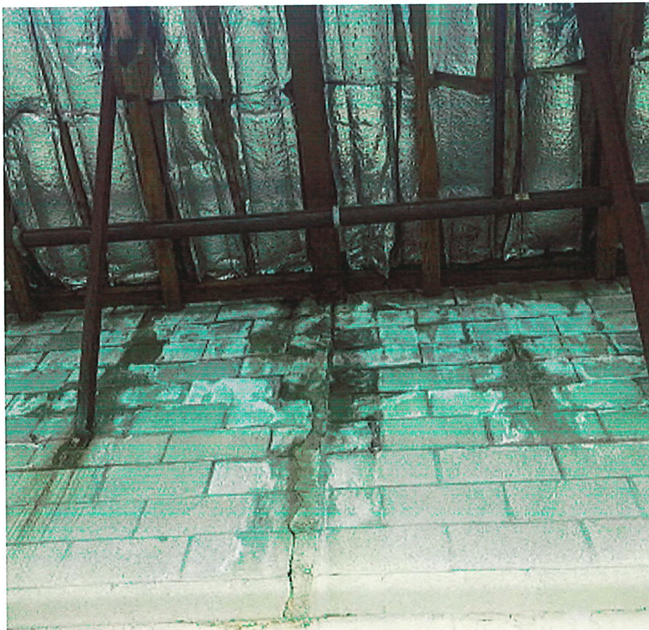
Photo 28 – Wall deterioration, Building C
