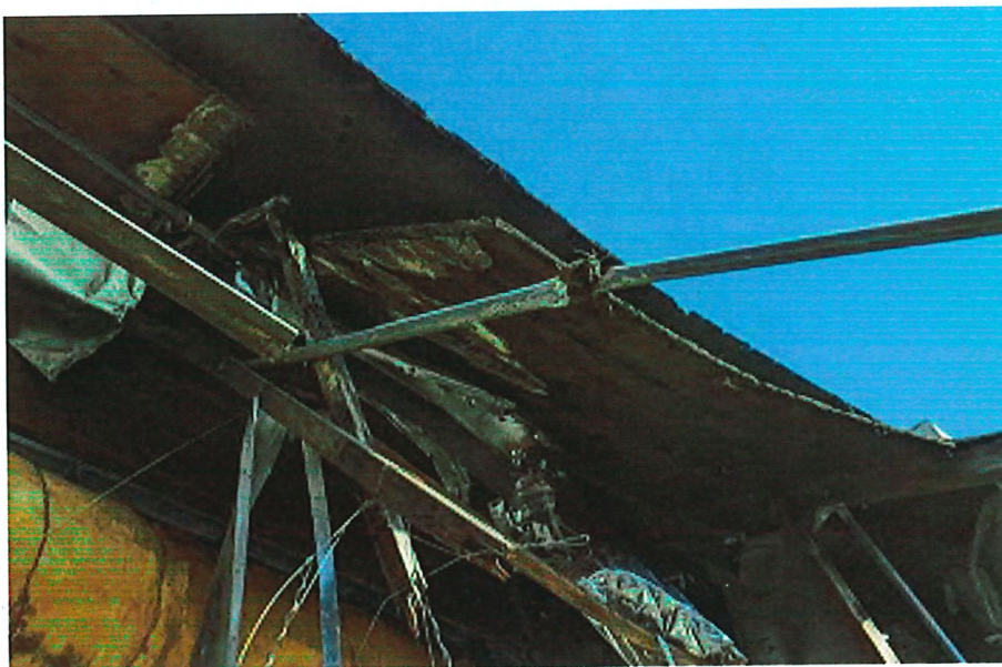
Photo 6 – Deteriorated top chord material visible on pin, Building A
