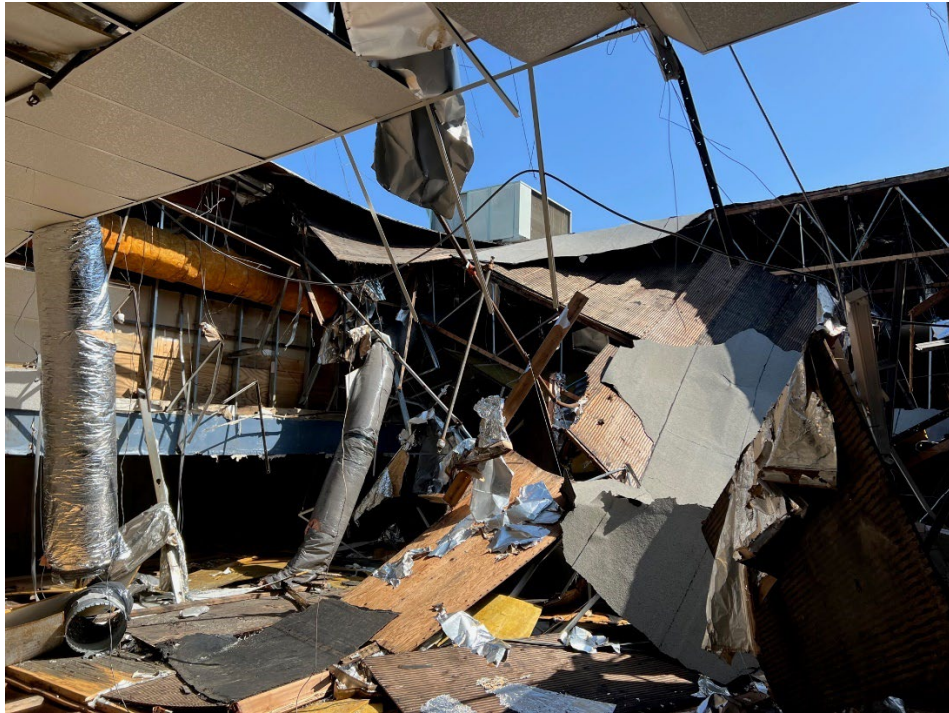
Unit A - Roof Collapse
