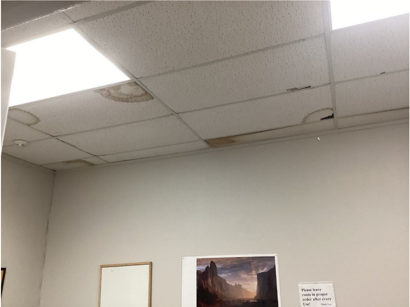
Units D – G 896/896a Lakeport Blvd. Multiple water markings on ceiling tiles
