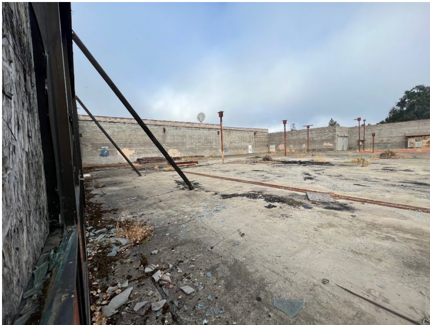
Unit B – Freestanding walls post initial roof collapse
