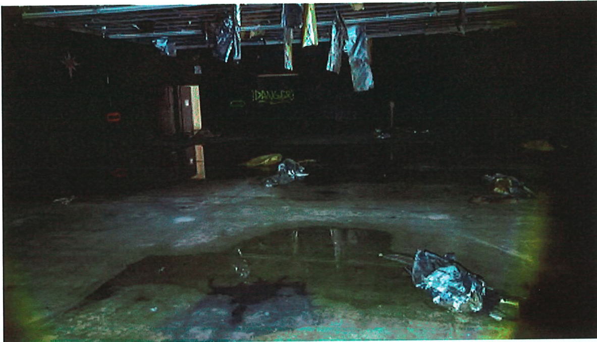
Photo 15 – Water collection at floor, Building A
