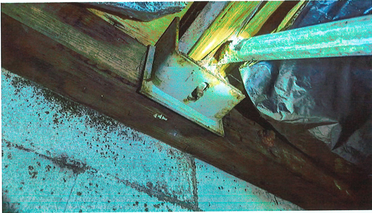
Photo 29 – Evidence of previous water intrusion, Building D
