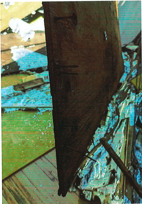
Photo 10 – Corroded nail withdrawal, Building A
