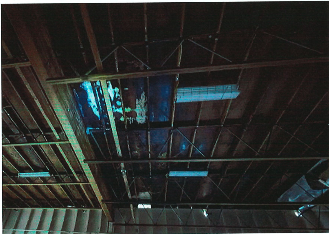
Photo 16 – Framing deterioration, Building A
