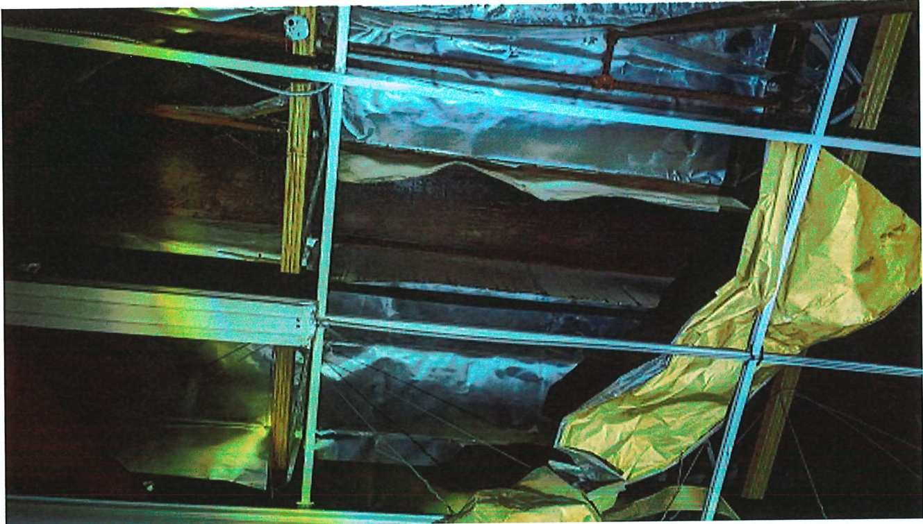
Photo 13 – Saturated framing, Building A
