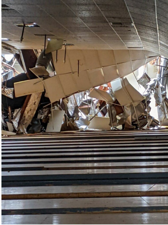
Unit A - Roof Collapse
