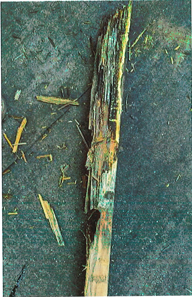
Photo 5 – Deteriorated truss top chord with pin bearing failure, Building A
