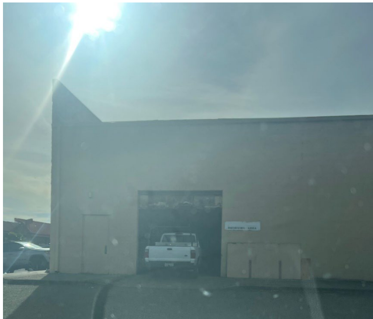
Unit A – Unpermitted demolition to enable vehicles to enter into the building
