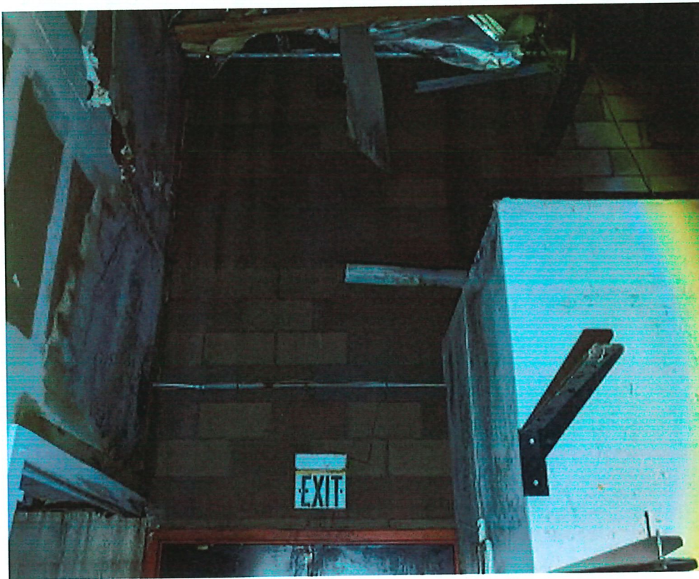
Photo 20 – Saturated back wall, Building A
