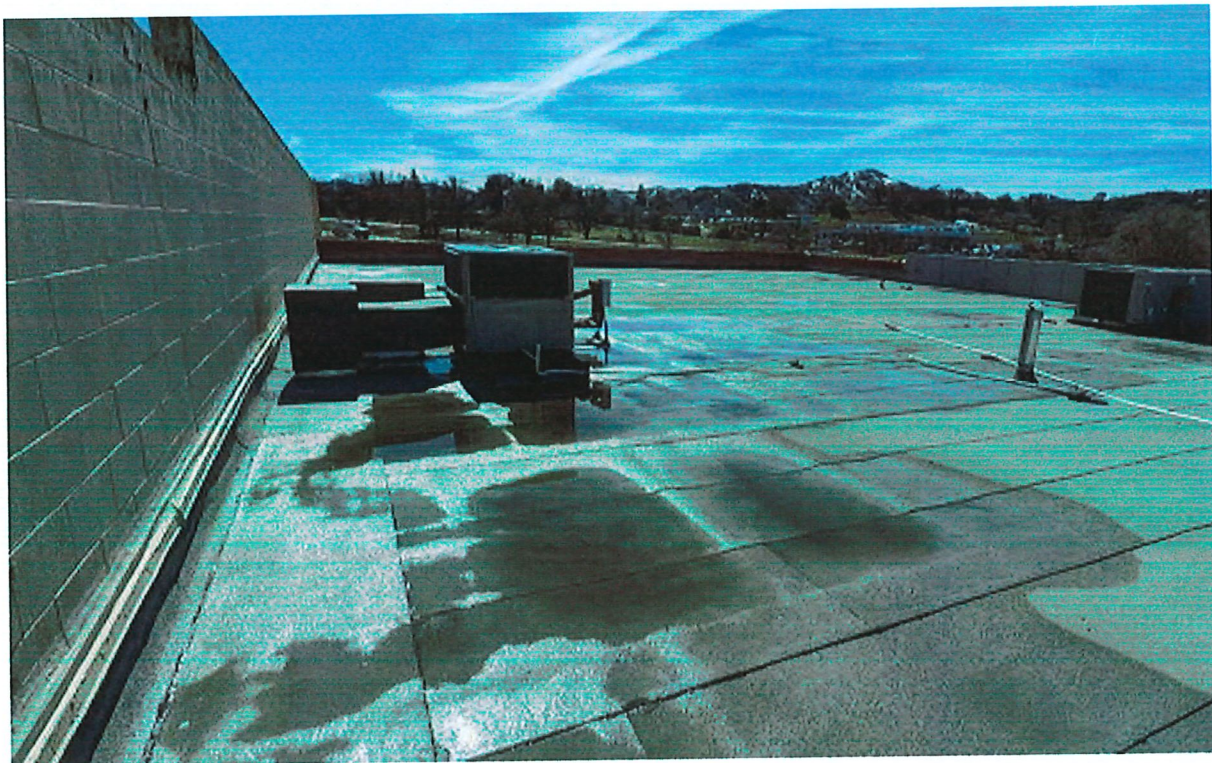
Photo 32 – Ponding at roof, Building D
