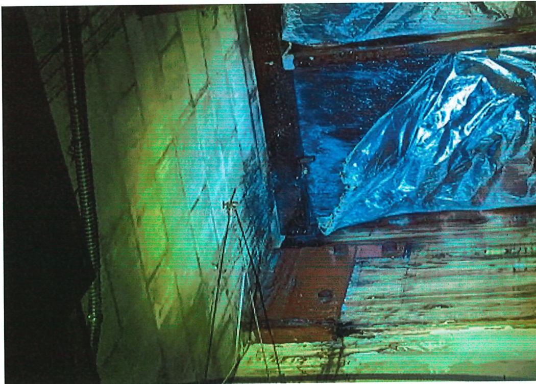
Photo 18 – Glulam beam deterioration, Building A
