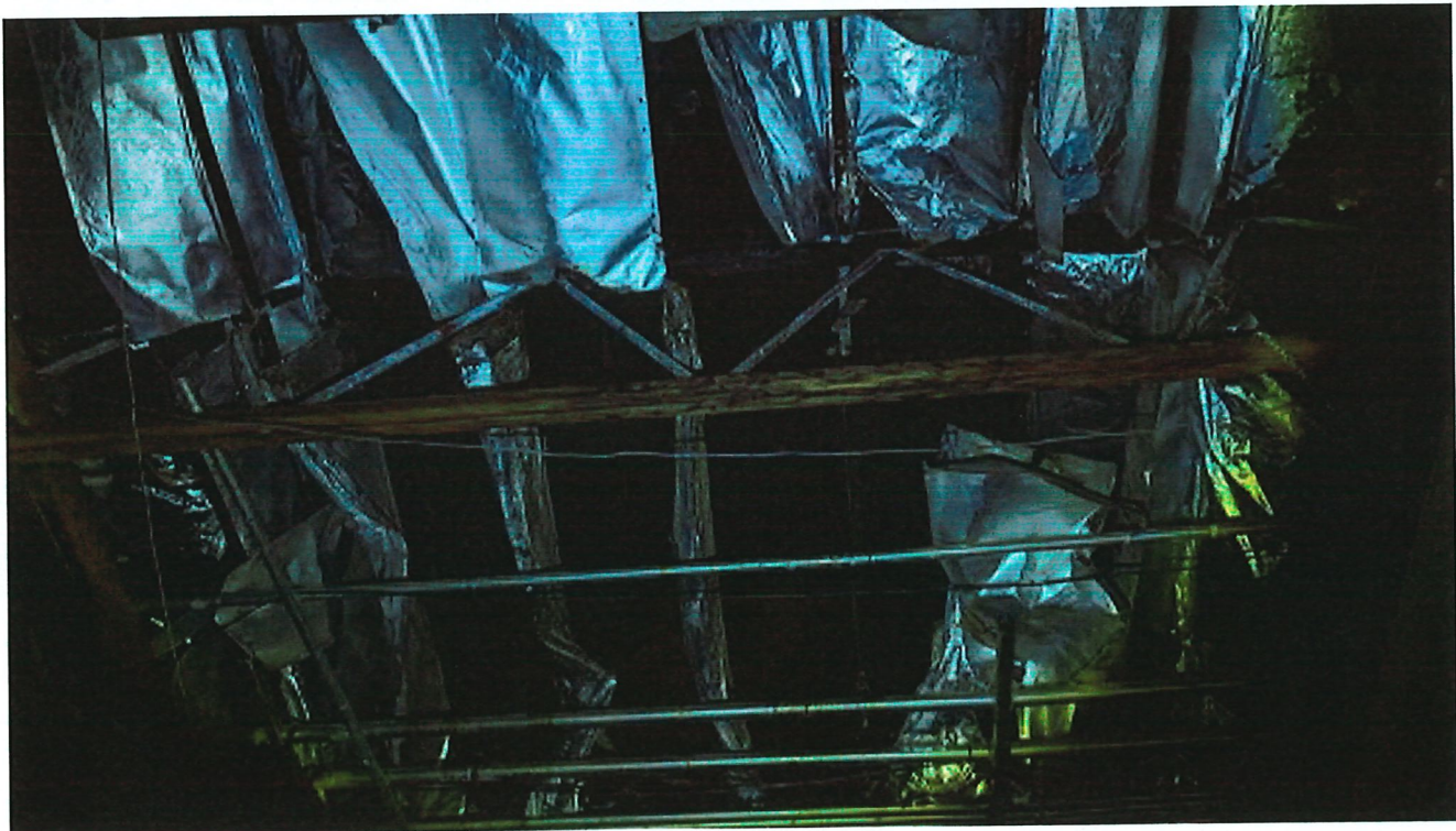
Photo 14 – Saturated framing, Building A
