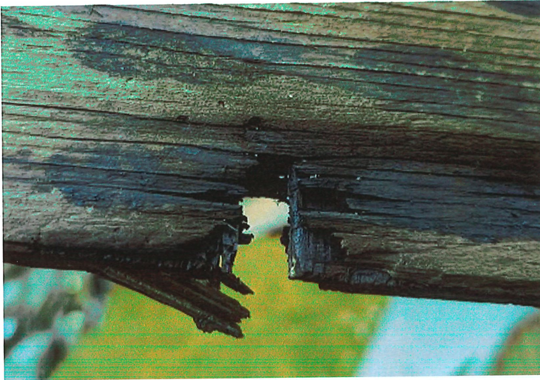
Photo 9 – Plywood nail edge distance failure, Building A
