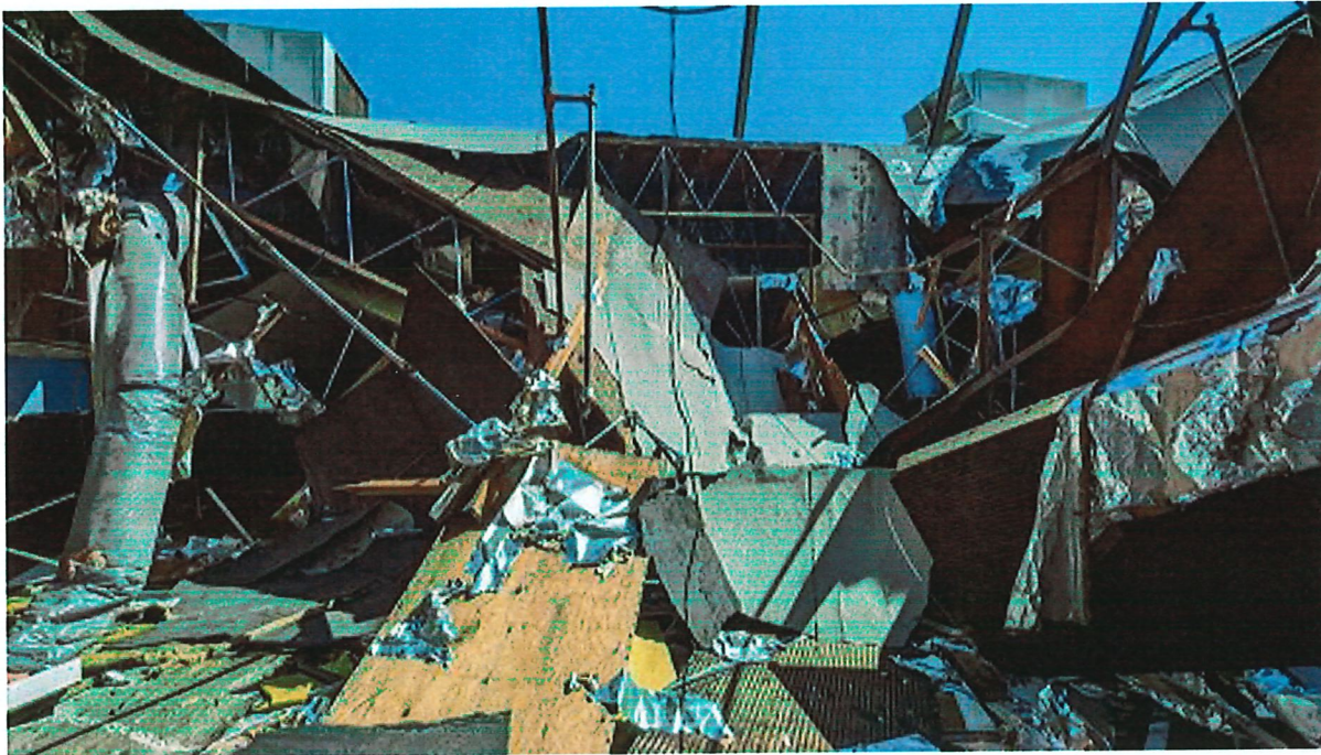
Photo 2 – Collapsed Roof, Building A
