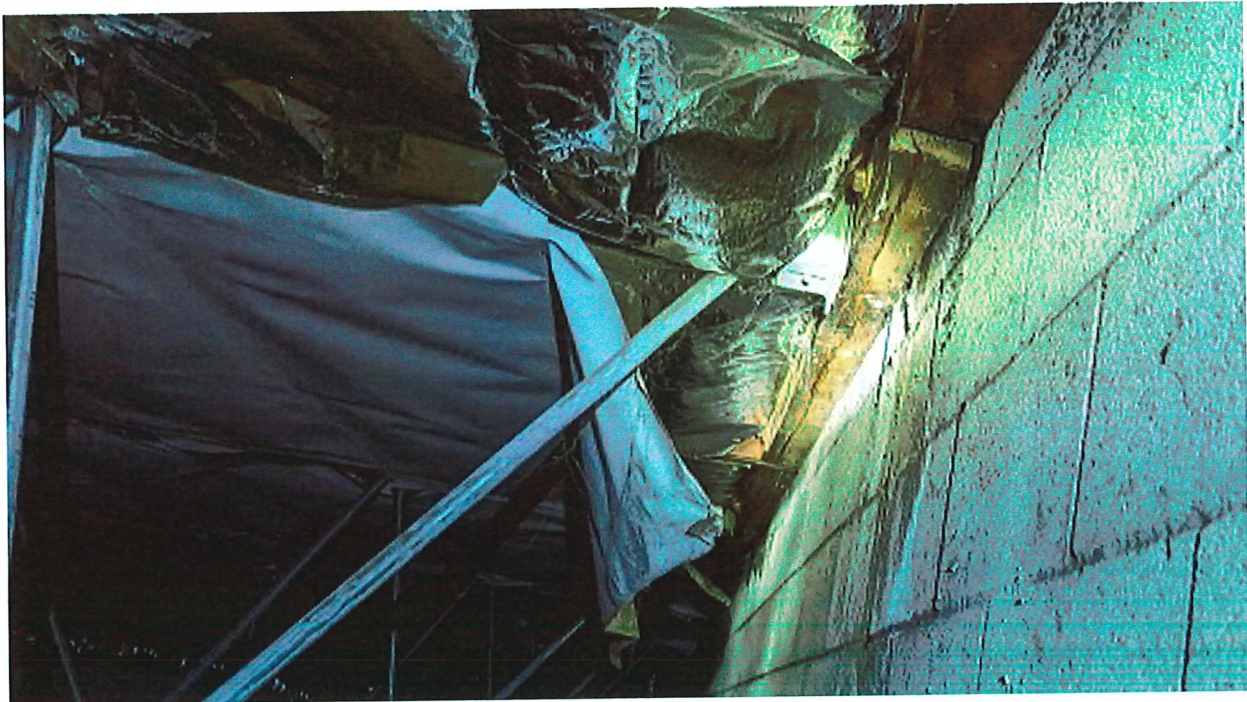
Photo 31 – Efflorescence at shared wall, Building D
