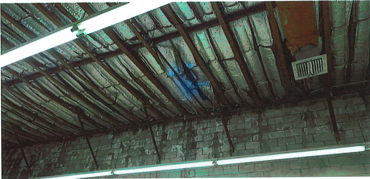
Photo 27 – Roof framing obstructed by insulation, Building C
