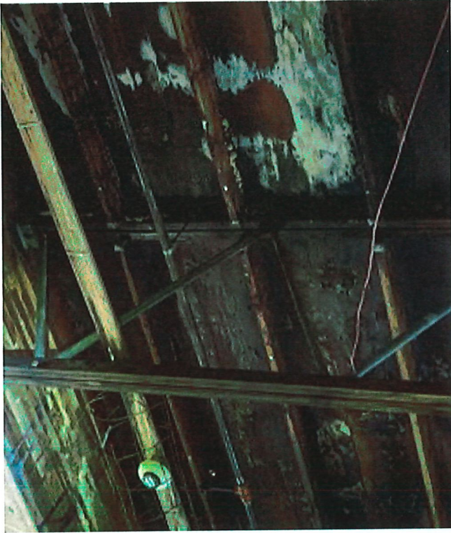
Photo 17 – Framing deterioration, Building A
