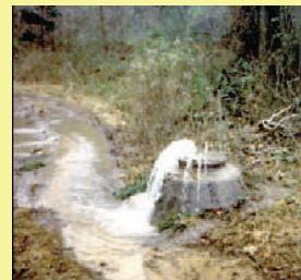
Example of a Sewer System Overflow (SSO)
