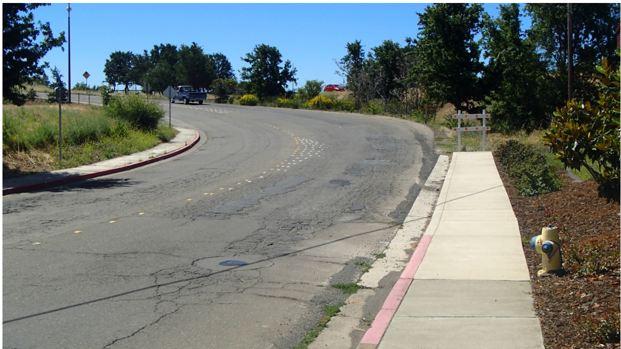
Figure 2: View to south along Bevins Street. Permitted parking due to lack of red curb and signing reduces southbound lane width to below standard.
