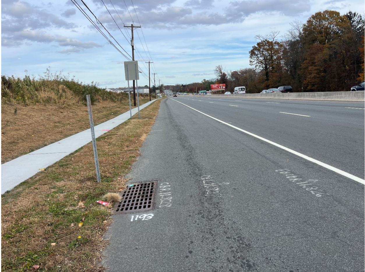
Photo 4: Photo facing east along the NJSH Route 38 frontage, showing open space/grass area.
