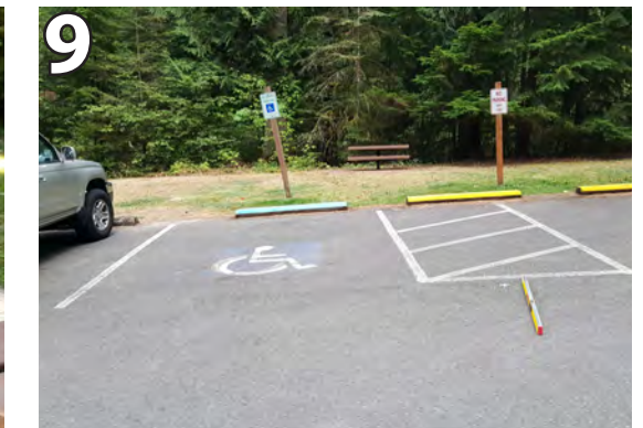
9 Running slope and cross slope of access aisle are not compliant. Install ADA compliant parking sign. (Sign has been removed since this picture was taken.)
