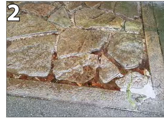
Excessive gaps and rise in flagstone entry. Reinstall so stones are level and gaps are no larger than 1/2".
