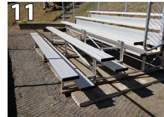
11 Bleachers not accessible. Install ADA compliant surfacing so that dugout, spectator area and field are flush
