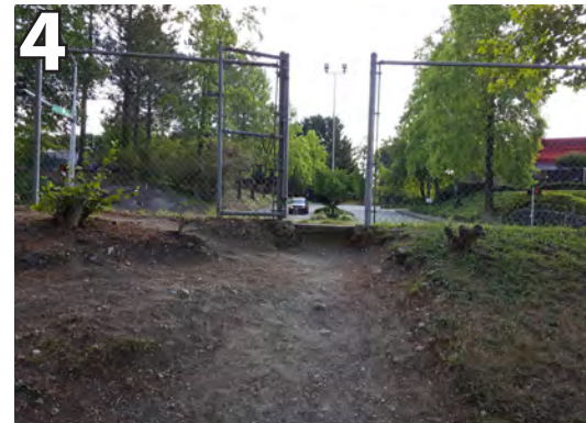
4 Park entrance not ADA accessible. Provide ADA accessible pathway that is flush with the sidewalk and connects to path below.
