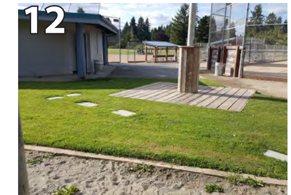
12 No accessible pathway to field #2. Install ADA compliant pathway.
