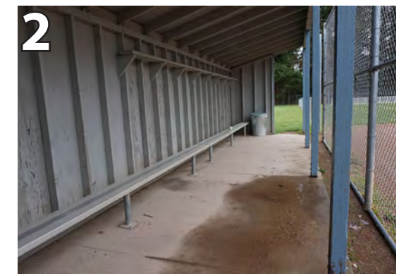
2 No wheelchair space in player seating for all 4 dugouts. Create opening that is centralized and at least 48" wide.
