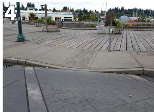
4 Curb ramp not ADA compliant. Regrade curb ramp.
