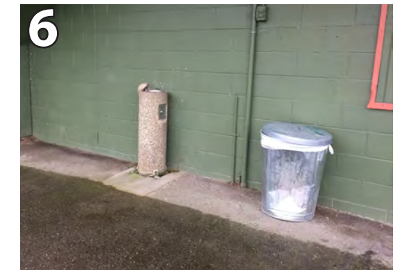
6 Non-compliant drinking fountain. Replace with ADA compliant drinking fountain.
