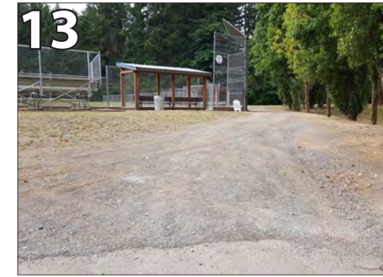
13 Non-compliant slope and surface. Re-grade to a slope no greater than 1:20 and replace surface with asphalt.
