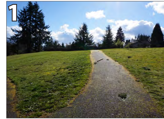
Running slope exceeds 5% and cross slope exceeds 2%. Regrade so pathway is ADA compliant.
