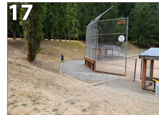
17 No ADA access to 3rd baseline dugout and spectator area. Replace surface w/ ADA compliant surface.
