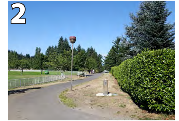
Drinking fountain is not compliant. Provide ADA compliant drinking fountain and relocate next to existing pathway.
