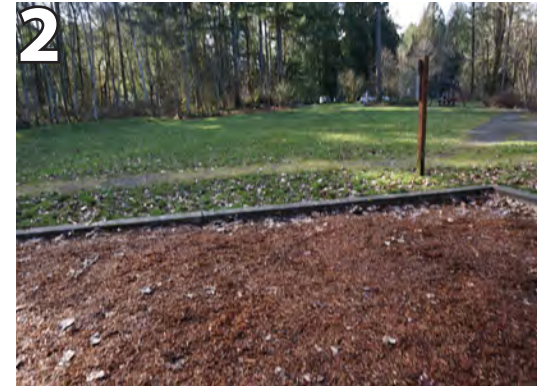
2 Provide ADA accessible ramp into swingset area.
