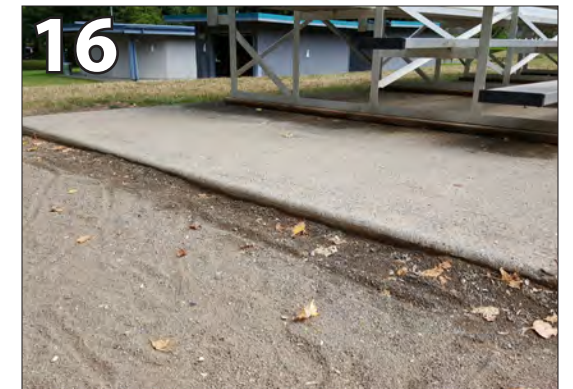
16 Spectator area not flush w/ crushed stone area.
