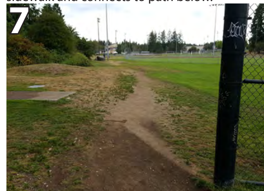
7 Pathway not ADA accessible. Install 60" ADA asphalt pathway.
