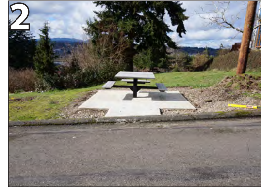
Provide curb ramp to allow for access to ADA accessible picnic table.
