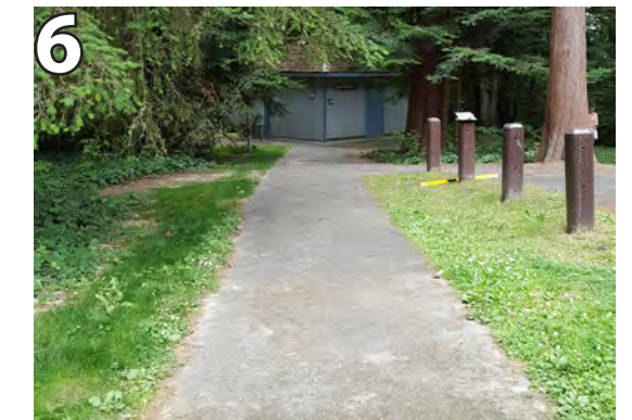
6 Running slope is greater than 1:20 and cross slope exceeds 1:48. Asphalt has surface bumps greater than 1/2". Regrade and resurface.
