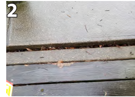
2"+ gap and 2"+ lift between sidewalk and overlook decking. Patch gap with concrete and shave sidewalk to be flush with decking.
