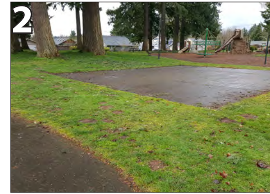
2 Provide ADA compliant pathway connecting trail to basketball court.
