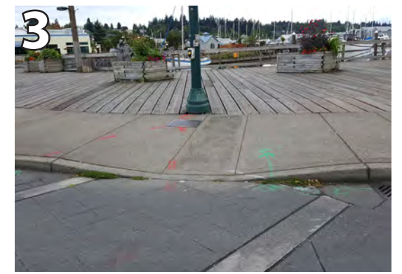
3 Curb ramp not ADA compliant. Regrade curb ramp.
