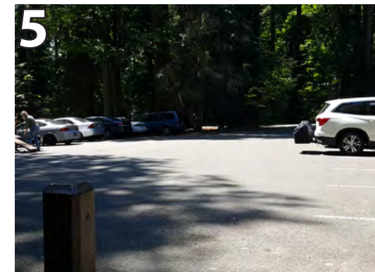
5 Inadequate ADA parking. Provide (1) ADA accessible parking space with proper signage
