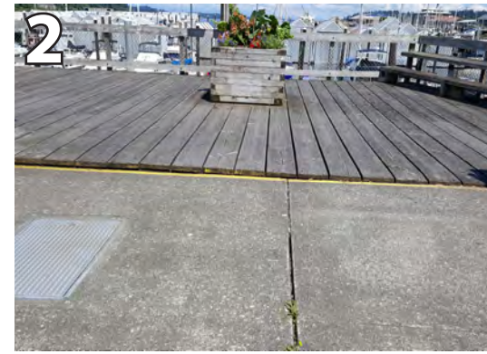
2 Entrance onto boardwalk to high. Regrade sidewalk to be flush.
