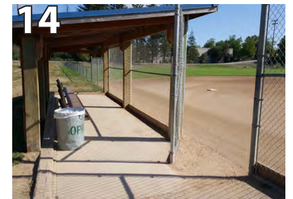
14 Inadequate space for wheelchair next to bench in dugout. Provide space that at least 36" x 48".
