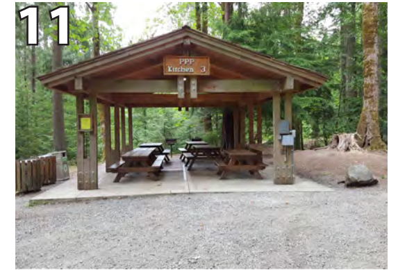
11 No ADA parking. Shelter threshold exceeds 1/2". Provide (1) ADA parking space. Install ADA pathway from ADA parking space to shelter.
