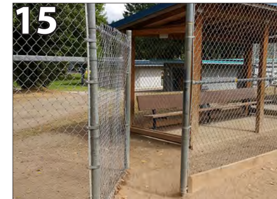
15 Fence opening too narrow. Widen to 36".
