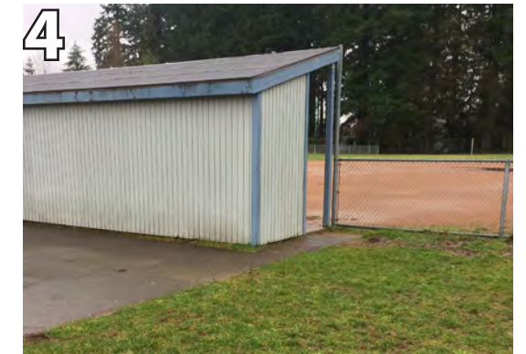
4 Pathway to dugout opening is too narrow. Widen to 60".
