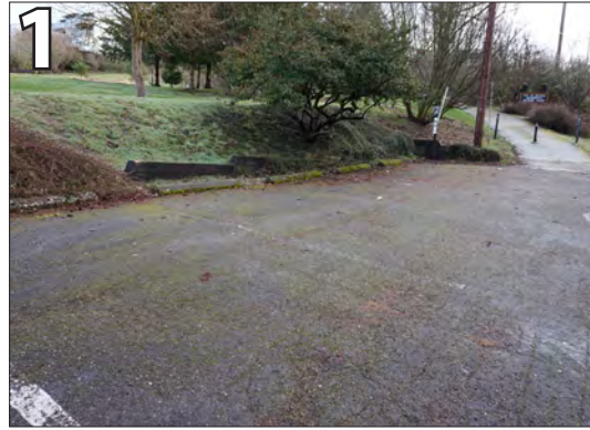
No ADA parking. Provide (1) ADA compliant parking space that has proper grade, markings and signage.
