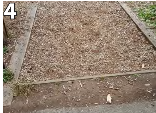
4 No ramp into engineered wood fiber play area. Install ADA accessible ramp into play area.
