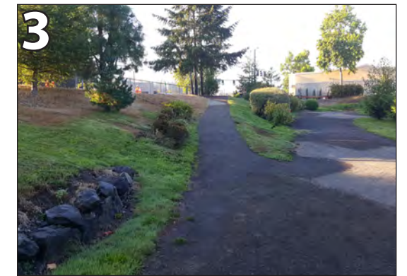
3 Pathway exceeds 1:20 slope and is considered a ramp. Install hand rails.
