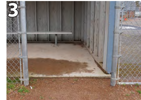
3 Thresholds of all but 1 dugout entrances exceed 1/4" in height. Grind down concrete so it is flush with field.
