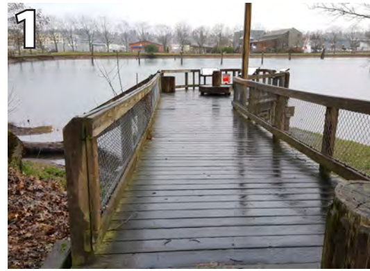
Decking is very slippery do to build up of moss. Implement a more frequent maintenance program or coat with anti-slip product.
