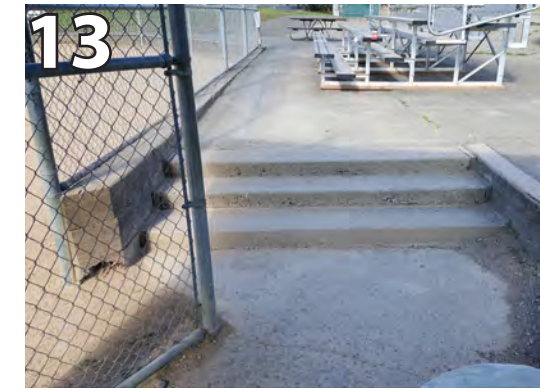
13 Dugout is not accessible. Provide ADA accessible ramp into dugout area.
