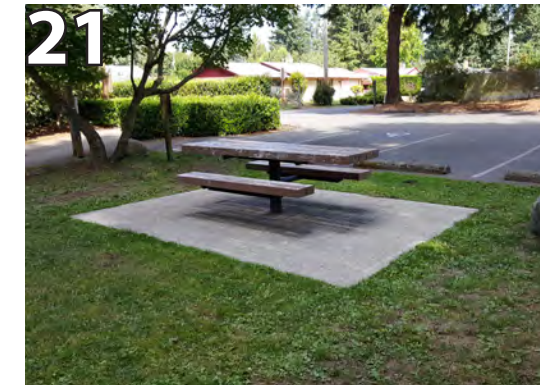
21 Picnic table not ADA compliant and is not accessible. Provide ADA accessible pathway to picnic table and install accessible picnic table.
