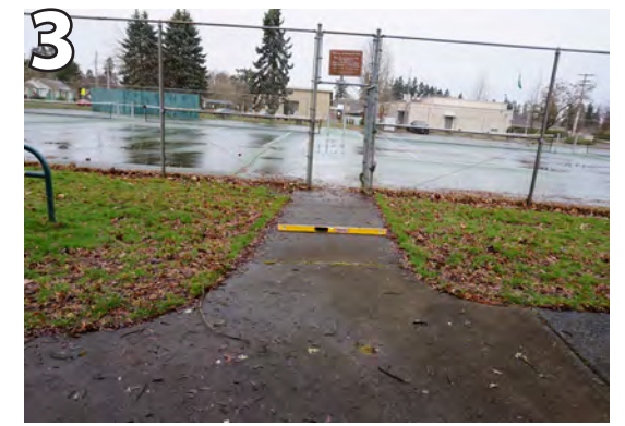
3 Pathway leading to tennis courts has a running slope of 6.6% and cross slope of 6.1%. Regrade pathway to be ADA compliant.
