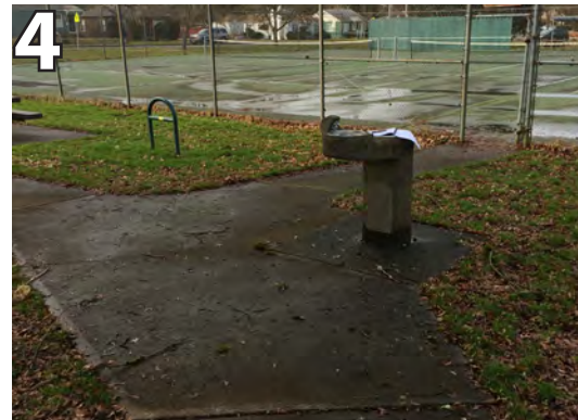
4 Non-compliant drinking fountain. Replace with ADA accessible drinking fountain.
