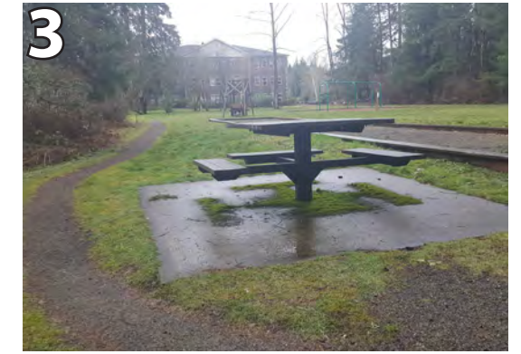
3 Picnic table pad not easily accessible. Provide a flush surface from pathway to concrete pad.
