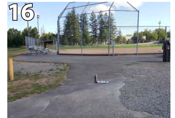
16 Running slopes and cross slopes are not compliant. Re-grade and resurface,
