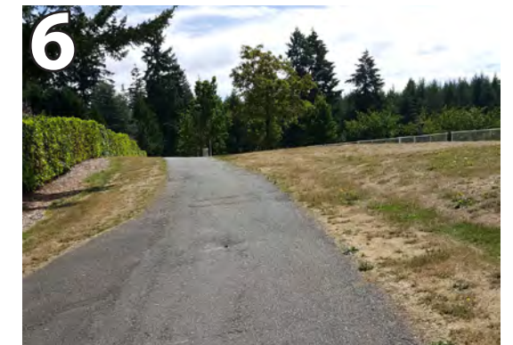
Exceeds 1:20 running slope and 1:48 cross slope. Regrade and repave.
