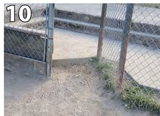
10 Transition from field to dugout exceeds 1/2". Grind concrete so field and dugout are flush.
