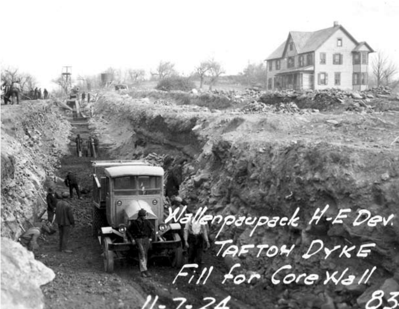
There's more to Wallenpaupack than meets the eye. This 1924 photo shows excavation for the impervious earth fill that has kept the Tafton Dike intact for more than six decades.
