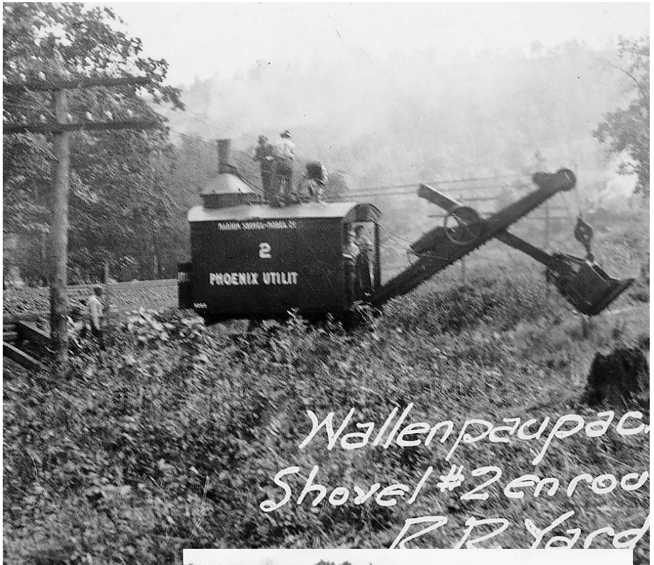
This steam shovel belonged to the Phoenix Utility Co., the builder of the Wallenpaupack project and the forerunner of PPL's Construction Department.
