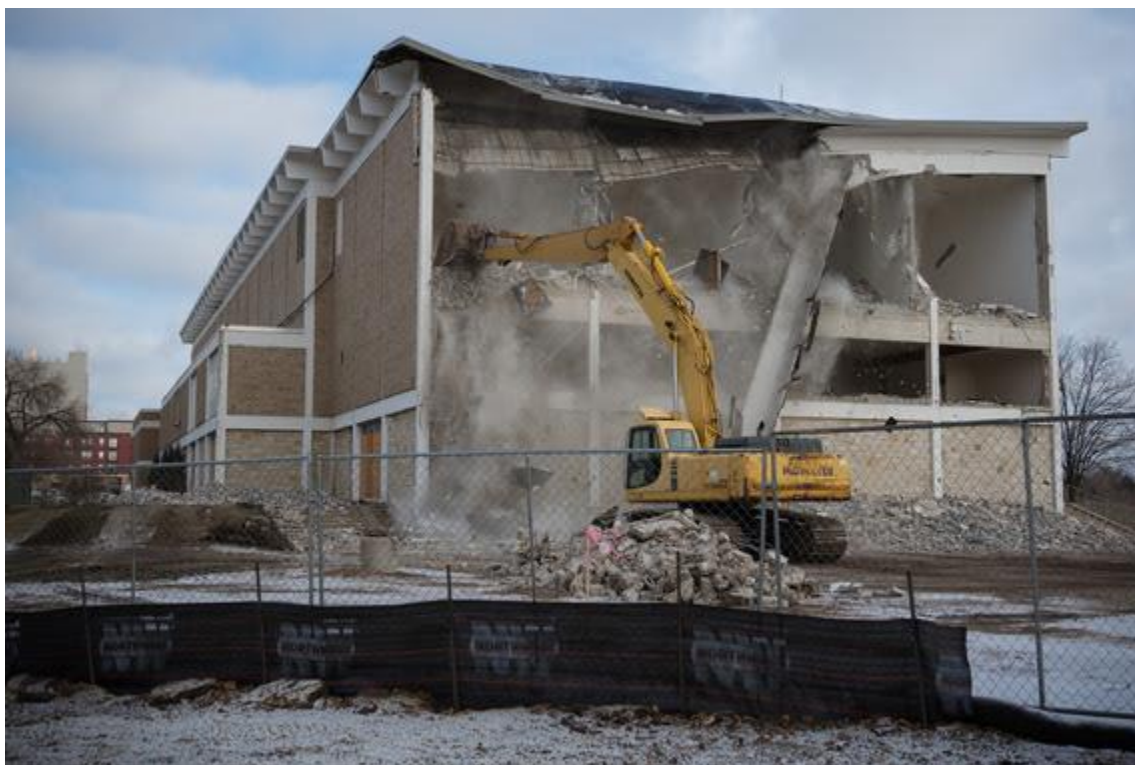
An excavator tears down a wall at the YMCA; photo credit: Joe Ahlquist / Post Bulletin
