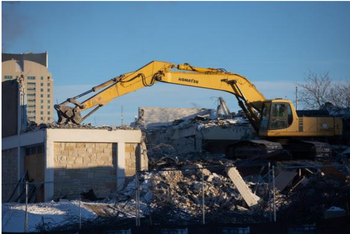
An excavator salvages recyclable material at the YMCA; photo credit: Joe Ahlquist / Post Bulletin
