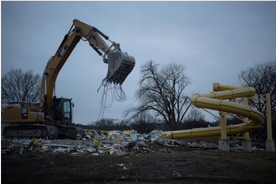
An excavator salvages recyclable material at the YMCA; photo credit: Joe Ahlquist / Post Bulletin
