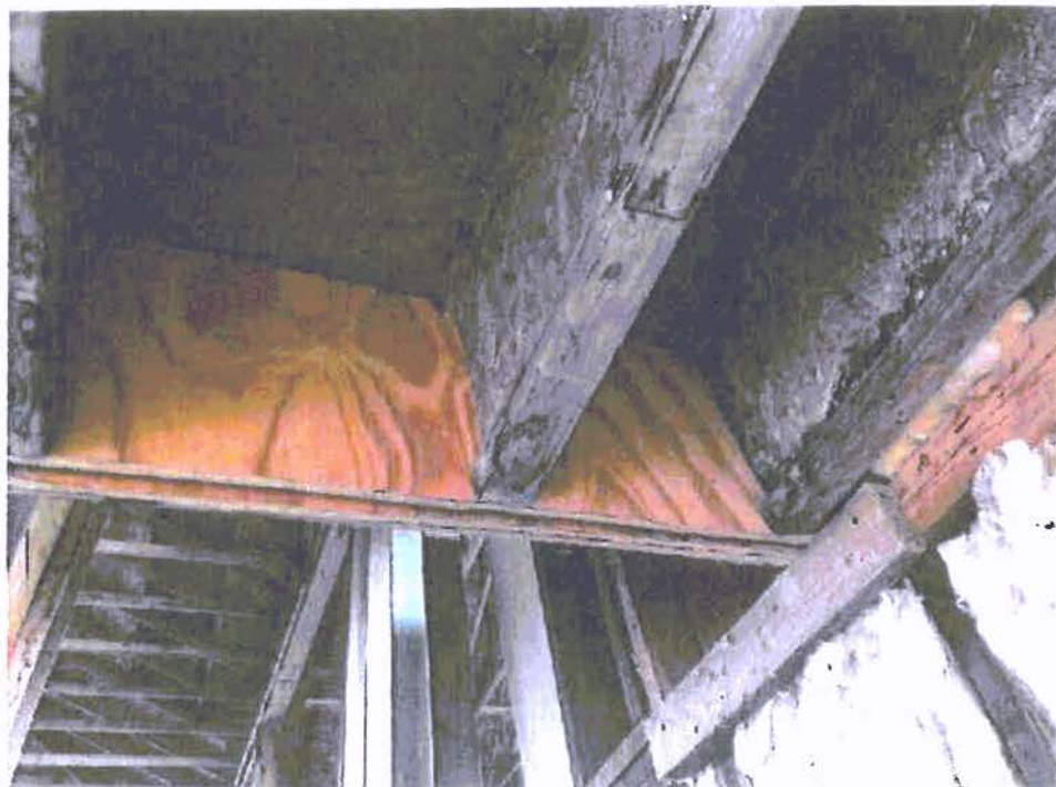
A-74: RIGHT SIDE OF HEADER, NO HANGERS PRESENT
