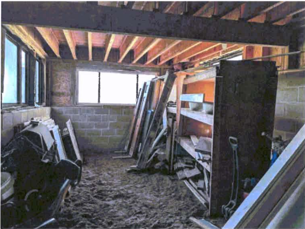
Photograph 1: Missing basement floor slab (2022).
