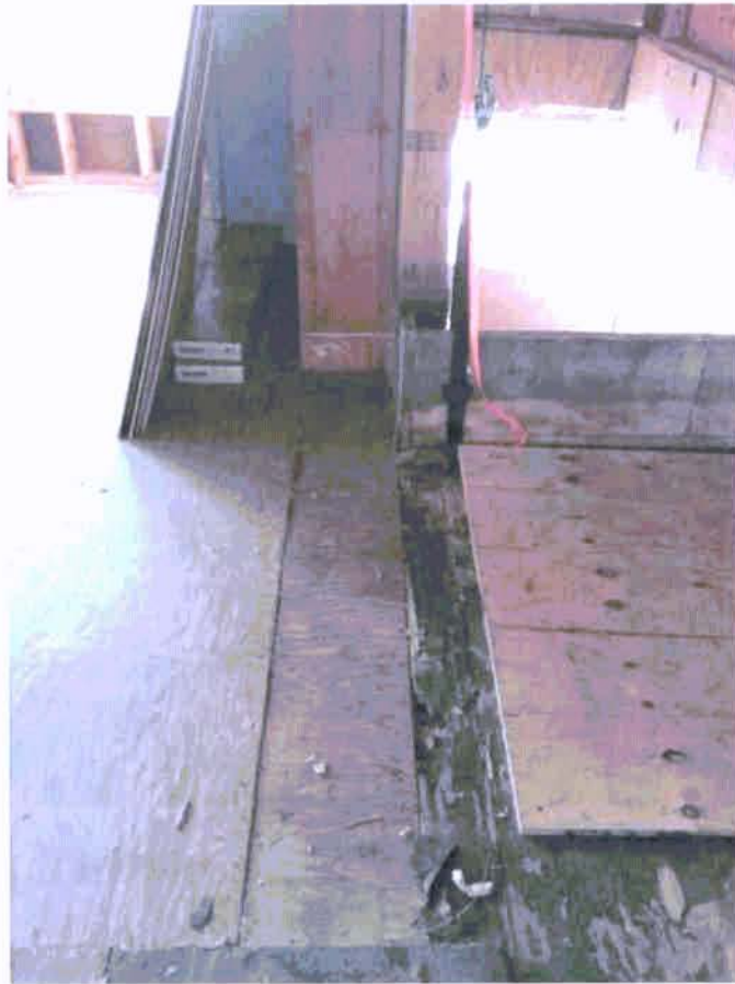
Photograph 11: Water damage on flooring (2022).
