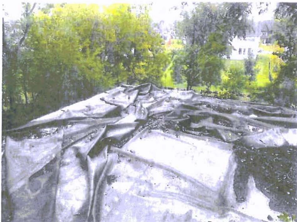
A-32: VIEW OF LOOSE MEMBRANE OVER PORCH
