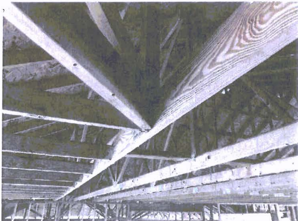
A-36: NO HANGER AT WEST HIP FRAMING
