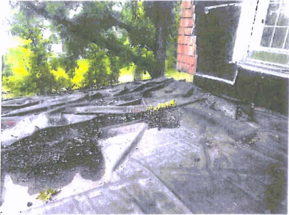
A-33: LOOSE MEMBRANE OVER PORCH
