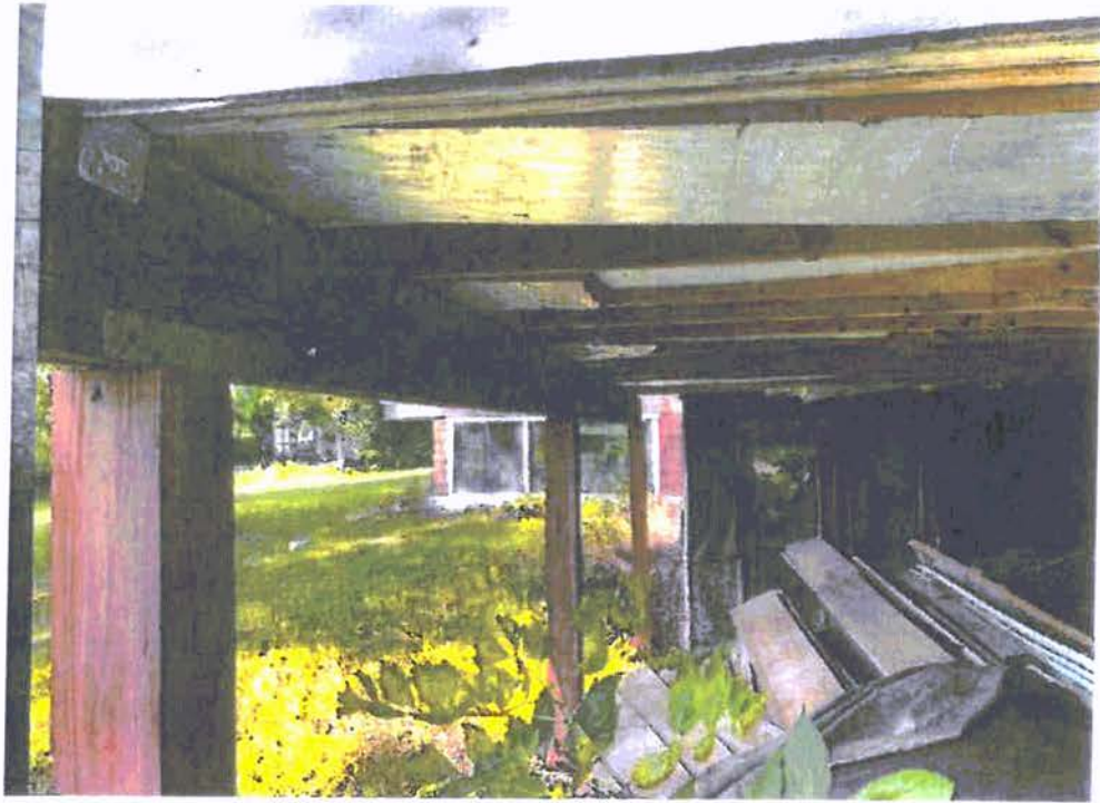
A-91: VIEW OF CRIB WALL UNDER EAST SIDE OF ORIGINAL PORTION OF HOME
