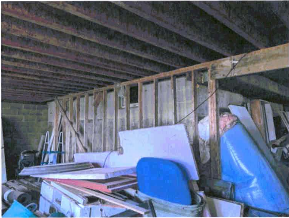
Photograph 15: Missing mid-height blocking on bearing wall (2022).
