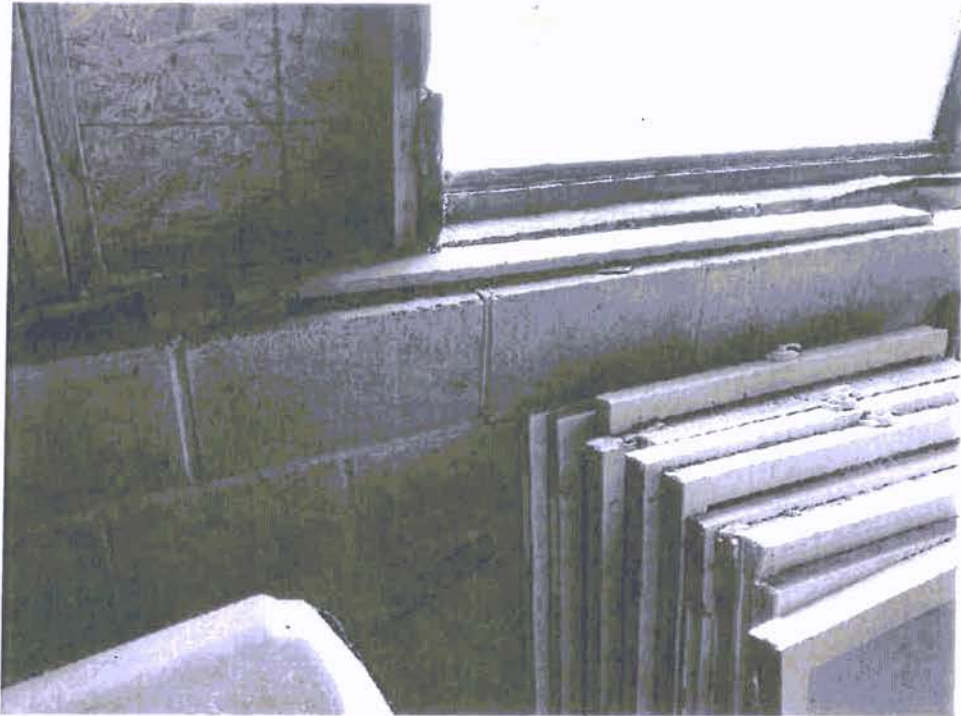
A-81: AREA WITH CRACK IN MASONRY BLOCK, EAST WALL, SOUTHWEST QUADRANT
