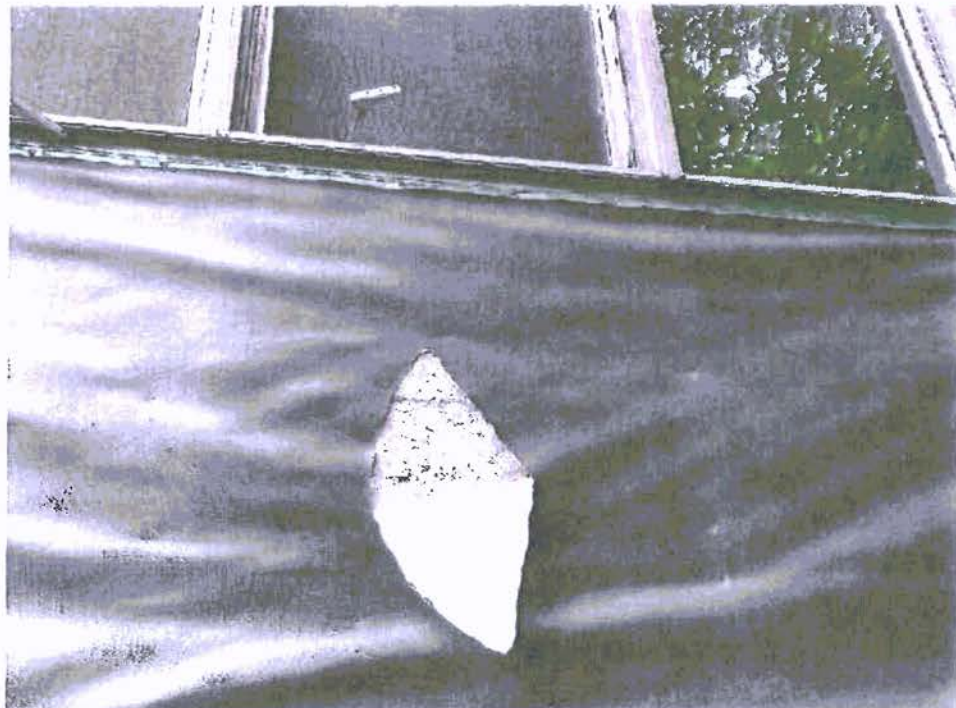
A-10: AREA OF SHEATHING EXPOSED AT EAST SIDE OF PORCH
