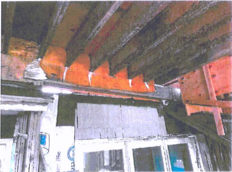
A-60: VIEW OF HEADER ALONG SOUTH SIDE OF ORIGINAL PORTION OF HOME
