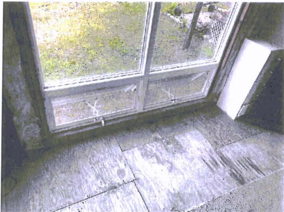
A-64: BASE OF WINDOW IN SOUTH WALL AT SOUTHWEST QUADRANT
