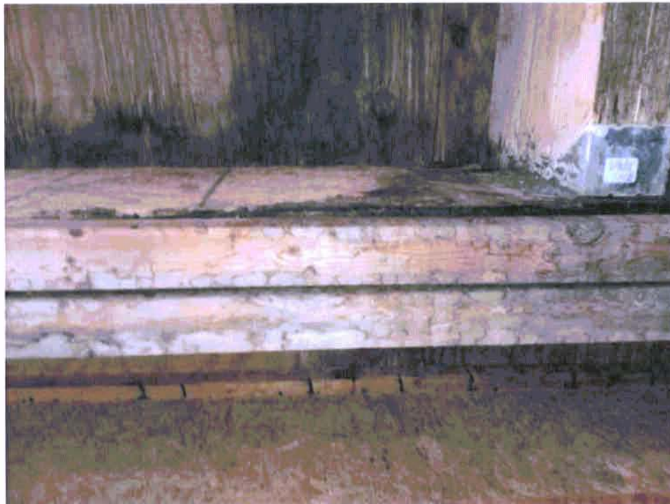
Photograph 12: Water damage on wood beams (2022).
