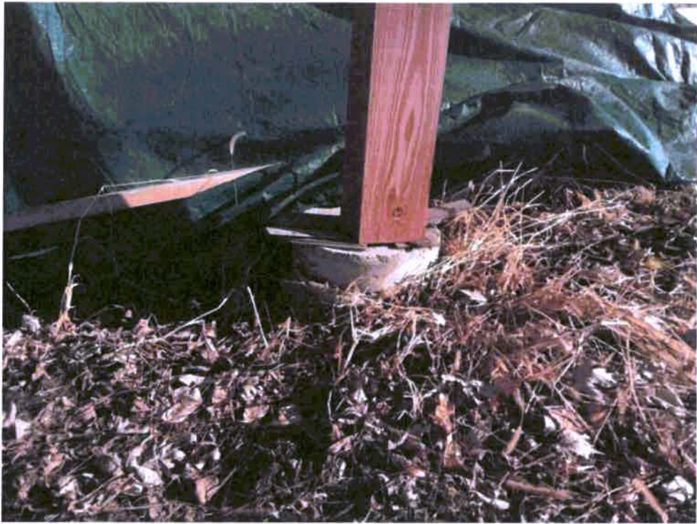
Photograph 9: Unaligned and unconnected post (2019).
