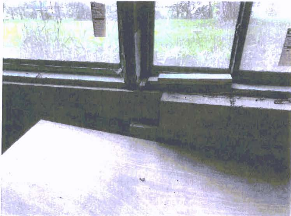
A-82: SHIFT IN FOUNDATION BLOCK, SOUTH WALL AT CENTRAL QUADRANT
