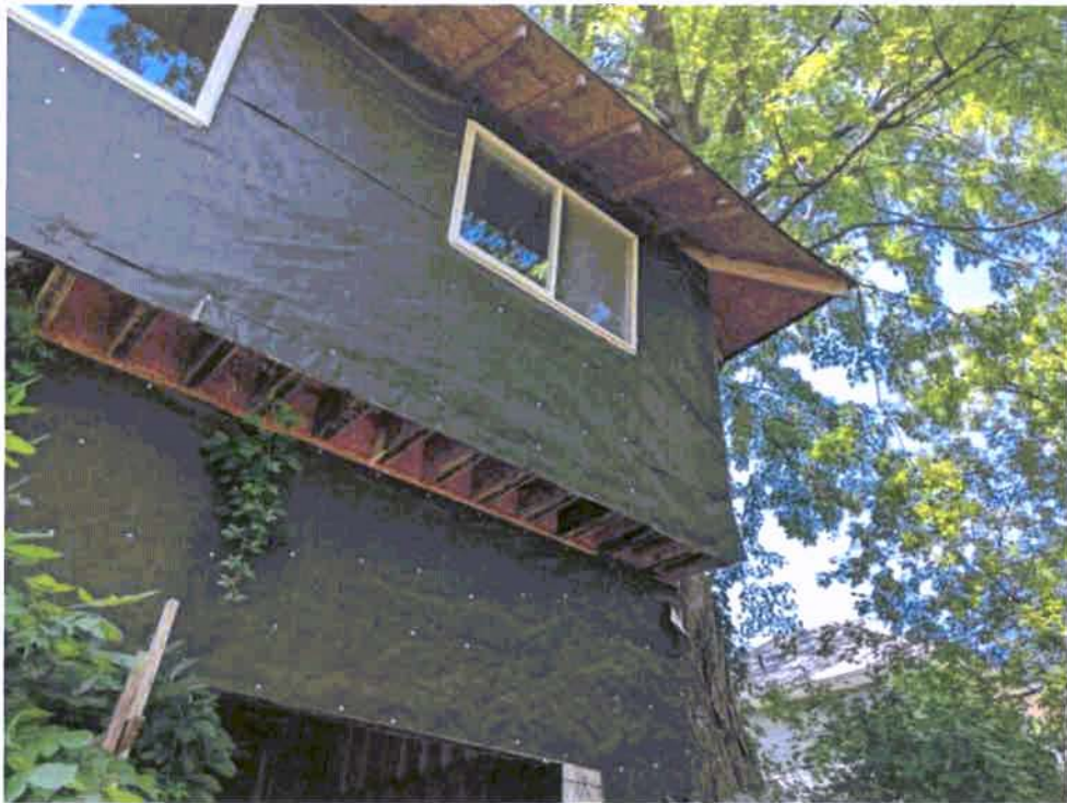
Photograph 5: Exposed soffits along exterior addition showing moisture damage (2022).
