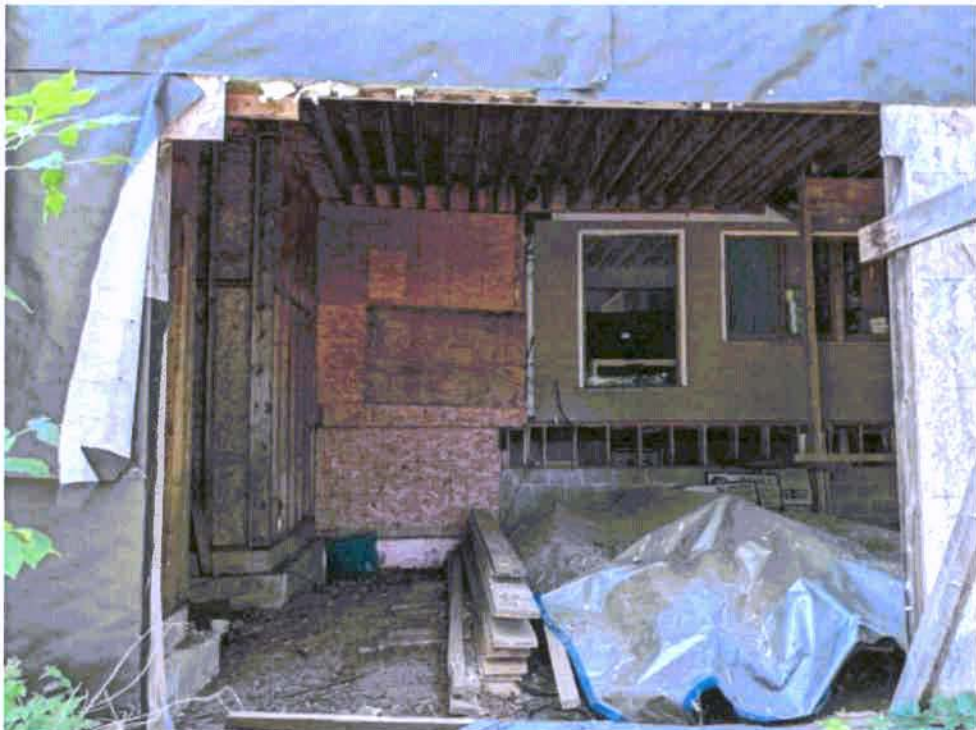
Photograph 2: Missing garage slab (2022).
