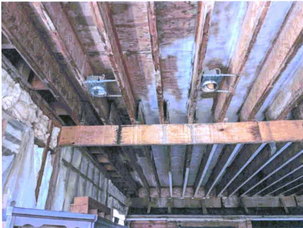
Photograph 4: Water damage and TJI beams (2022).
