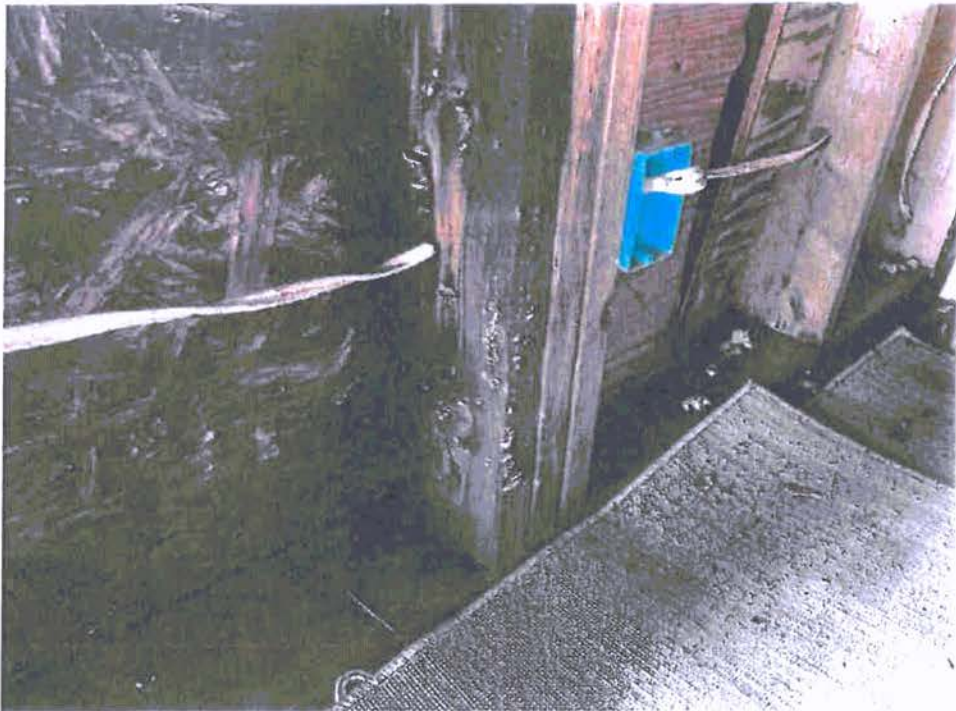
A-72: VIEW OF SHEATHING AND STUDS BELOW RIGHT SIDE OF SOUTH WINDOW
