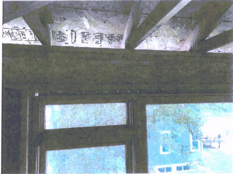
A-37: VIEW OF TOP OF WEST WINDOW IN NORTH WALL, FLANGE VISIBLE
