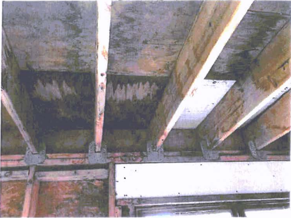
A-71: SOUTH WALL ABOVE LEFT SIDE OF WINDOW
