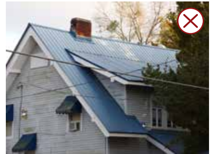
A brightly colored metal is an unacceptable roof replacement material.
