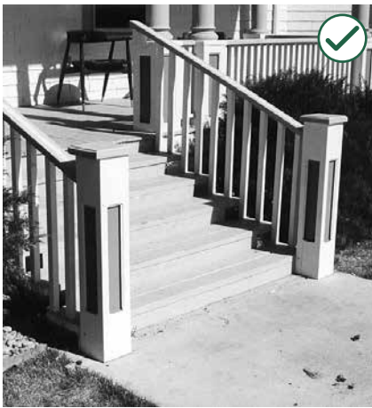
After: Railing has been repaired and the base of the post has been replaced in-kind. This is an appropriate approach.
