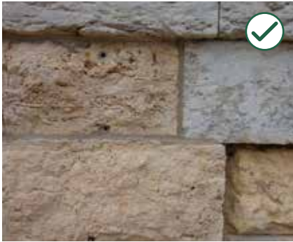
Preserve the historic wall materials of a building. The repointing in the bottom image is an appropriate and needed treatment.
