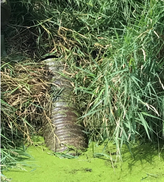
Figure 2: Deteriorating, submerged outlet
