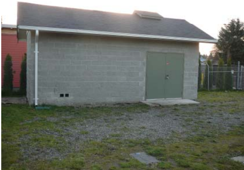
Figure 3: Well #1A Pumphouse
